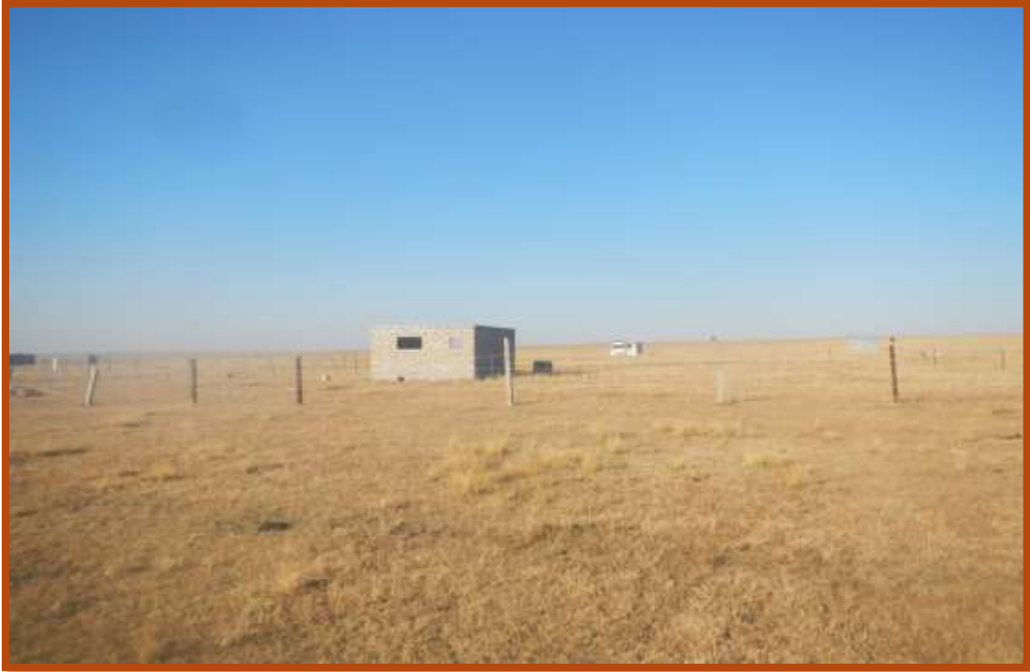
Figure 9: A partially built structure on the North Western side of the site
