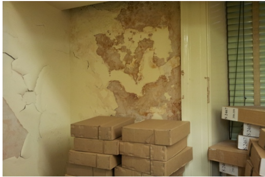
Raising damp & Leaks
