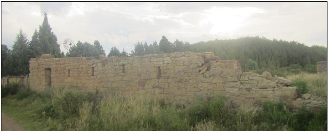
Figure 53: Ruined structure at the Bamboes railway station at waypoint 1887. Its function is unknown.
