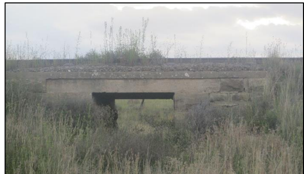
Figure 89: A railway bridge with stone walls and a concrete deck at waypoint 1786.
