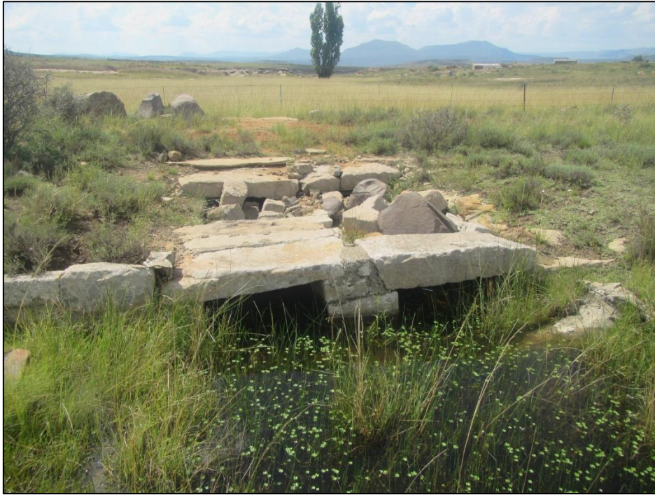
Figure 85: Small bridge built of stone slabs along the old district road at waypoint 1811. Some slabs have broken and caved in.
