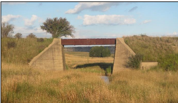
Figure 88: A railway bridge at waypoint 1636 with concrete walls and steel/cast iron deck.
