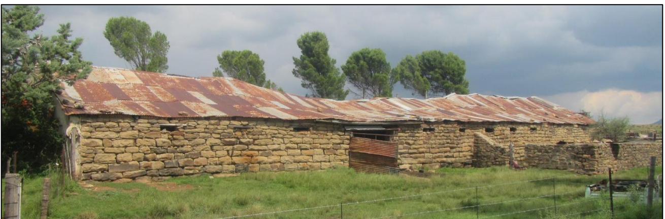
Figure 79: Stone-walled farm sheds at waypoint 1916. The sagging ridgeline shows that the roof trusses are collapsing.
