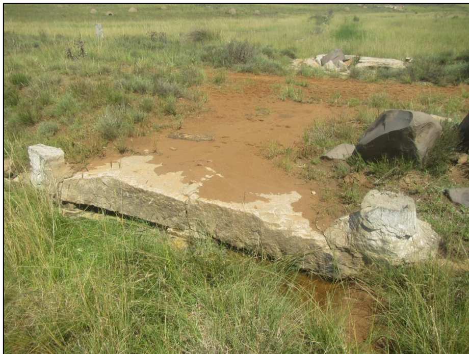
Figure 86: Opposite side of the bridge shown above (waypoint 1811). On the side of the left-hand slab in view is inscribed "GEBOU DEUR PJ COETZER".
