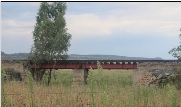
Figure 90: A railway bridge at waypoint 1787 with stone walls and central pillar and a steel/cast iron deck.
