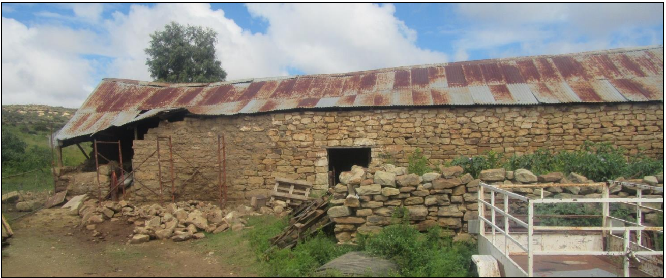
Figure 80: A stone-walled barn at waypoint 1957 whose end had recently collapsed and was being rebuilt using the same materials (stone and mud mortar).
