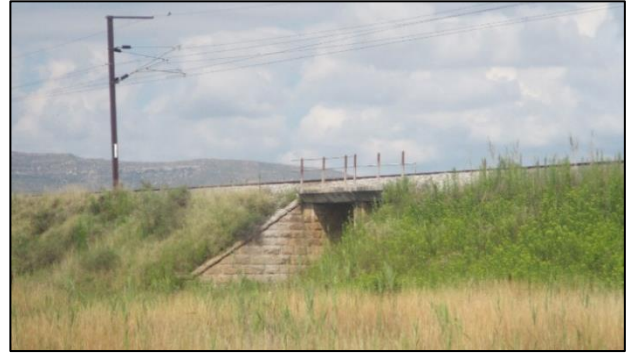
Figure 93: A railway bridge at waypoint 1794 with stone walls and pillar and a concrete deck.
