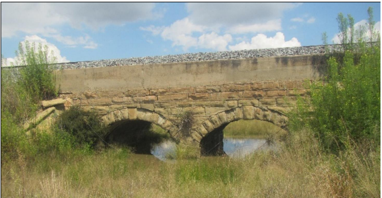
Figure 94: A stone railway bridge with arches at waypoint 1813. A concrete deck has been laid over the stonework. The wing walls are also of stone.
