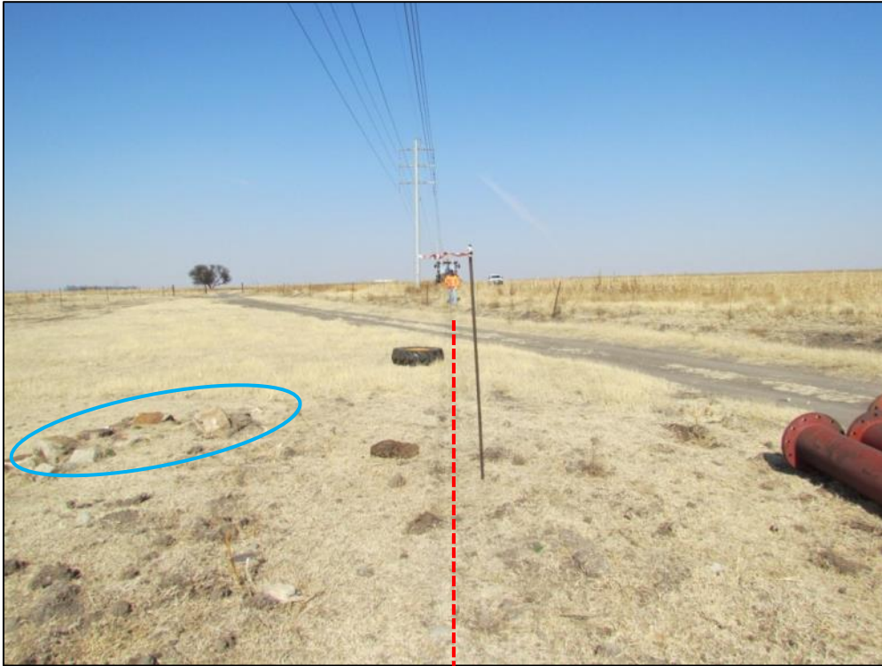
Figure 4-3: Sandstone foundation within pipeline route (red) before excavation. Note the location of the walls that will be temporarily buried (blue)
