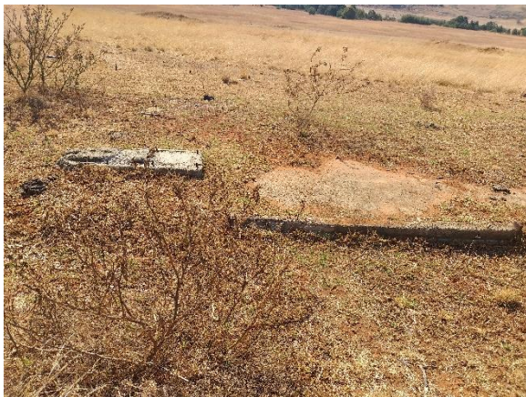
Example of a concrete foundation which may be associated with the historical built environment
