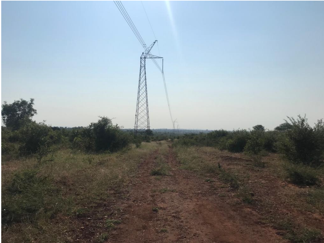
Figure 4: View of Eskom power line from Cahora bassa in Mozambique.
