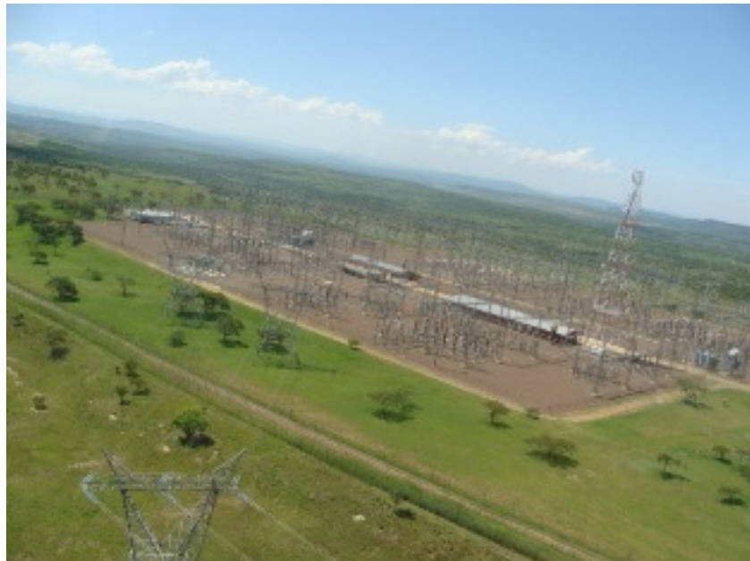
Figure 2: Venus substation from the air
