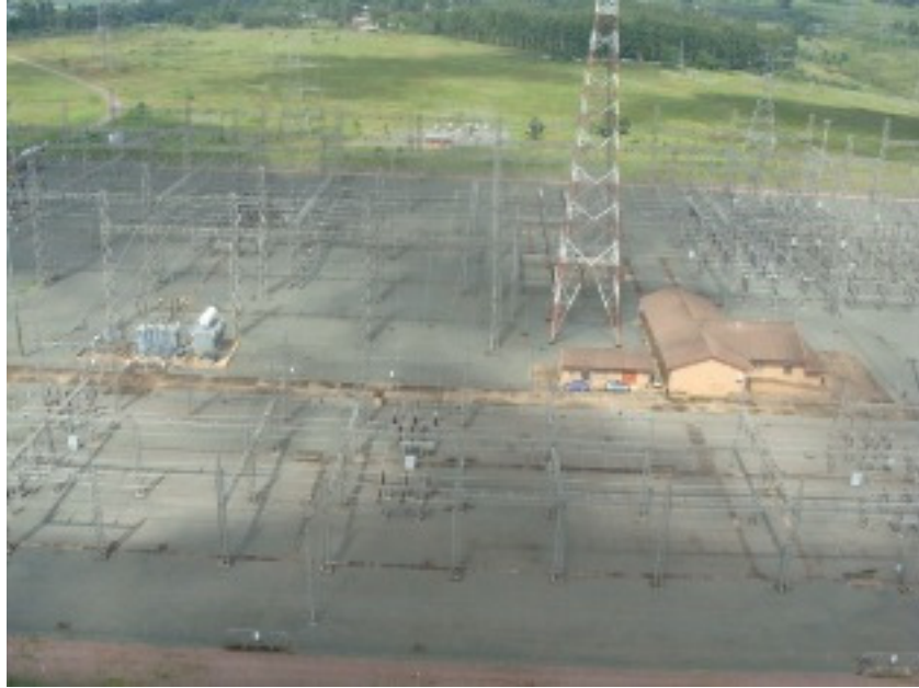
Figure 3: Ariadne substation from the air
