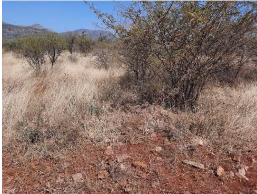
Figure 47 – Broken down foundation hidden among tall grass at Site 1-6
