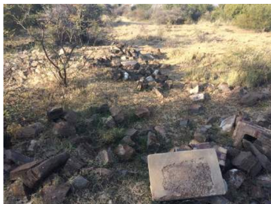
Figure 33 - Collapsed structure at site 023, showing a mix of constructive elements (concrete, bricks and cement).
