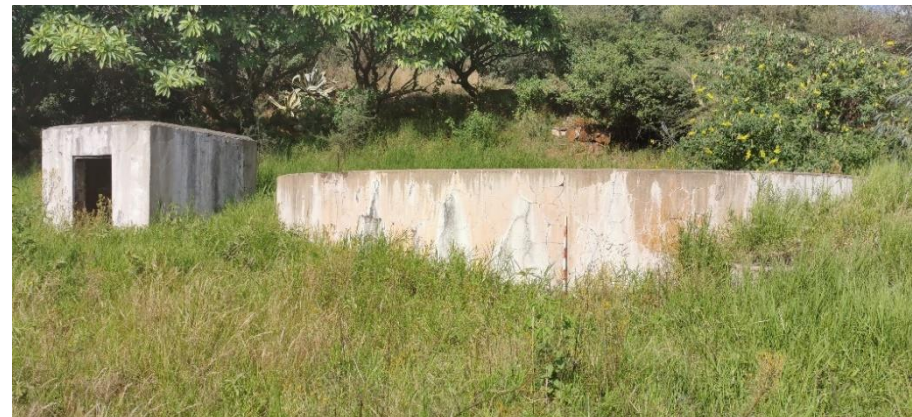
Figure 54 – General view of the small square structure and the possible reservoir located at site BFP-08. The scale is in 10cm increments.
