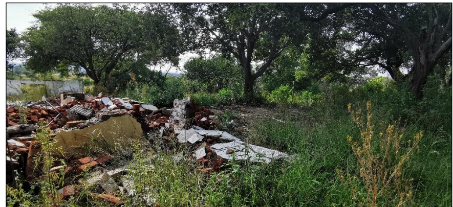
Figure 61 – General view of the rubble and broken-down structure located at site BFP-11.
