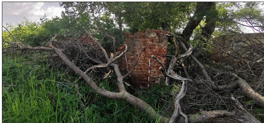
Figure 46 – General view of the small brick structure located at site BFP-04. The scale is in 10cm increments.
