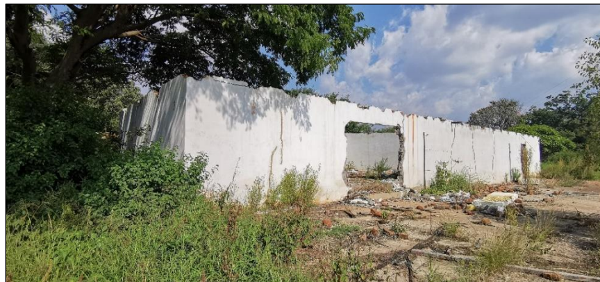
Figure 52 – General view of the structure located at site BFP-06. The scale is in 10cm increments.
