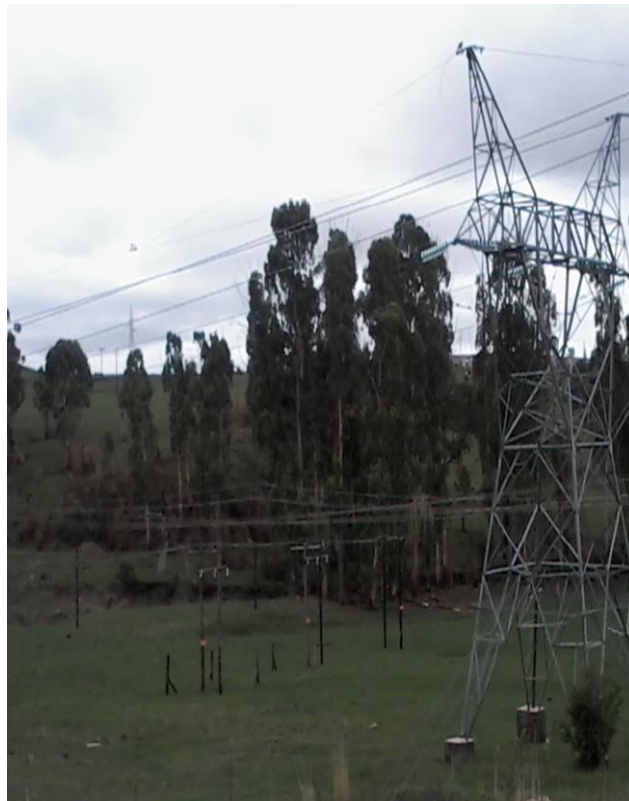
Photo #15: Powerlines in the vicinity of Vrede Substation
