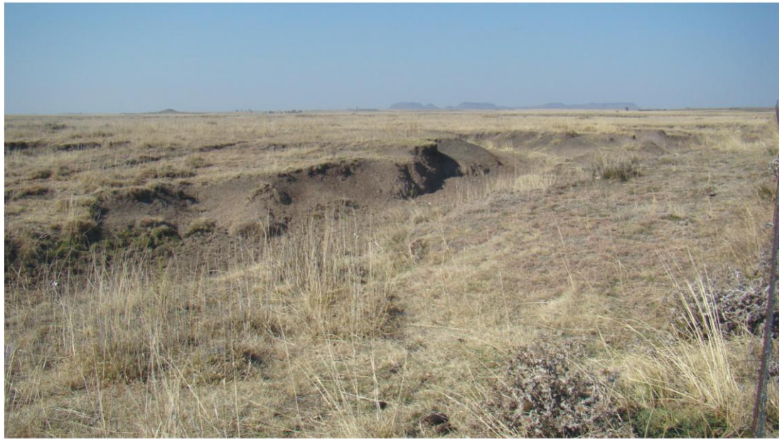
Figure 9. Rehabilitation of culverts will impact mainly on previously disturbed residual deposits and superficial deposits of Quaternary age.
