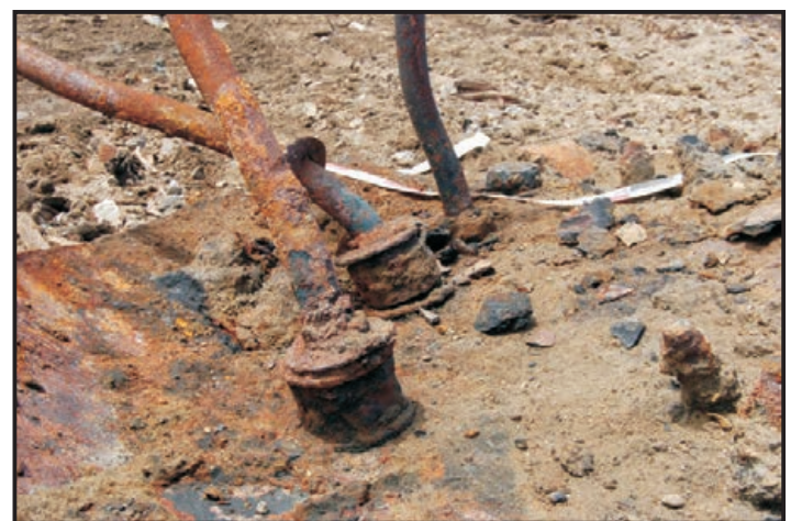
Figure 149: Close-up of the boiler stays on the inner surface of the boiler back plate (Photo: Maitland)
