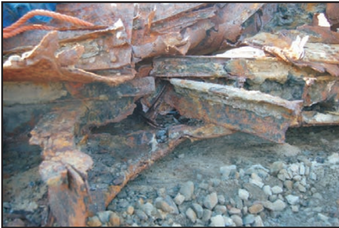
Figure 334: Keel showing centre keelson, intercostal keelson and reversed frames (Paasch 1890: Plate19; Photo: Maitland)
