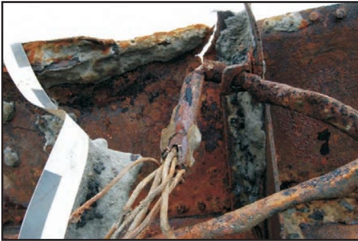
Figure 231: Electric wiring in a metal conduit (Photo: Maitland)
