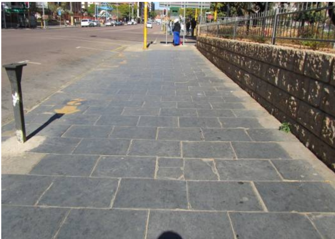
Figure 276. All street furniture has impact on paving. This now disused parking meter shows how not to implement and retire street furniture. (P 1074)
