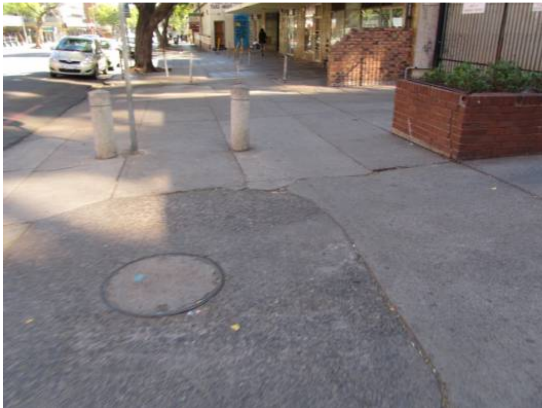
Figure 118. 'Concrete strip interruption in cement block paving. (P 917).
