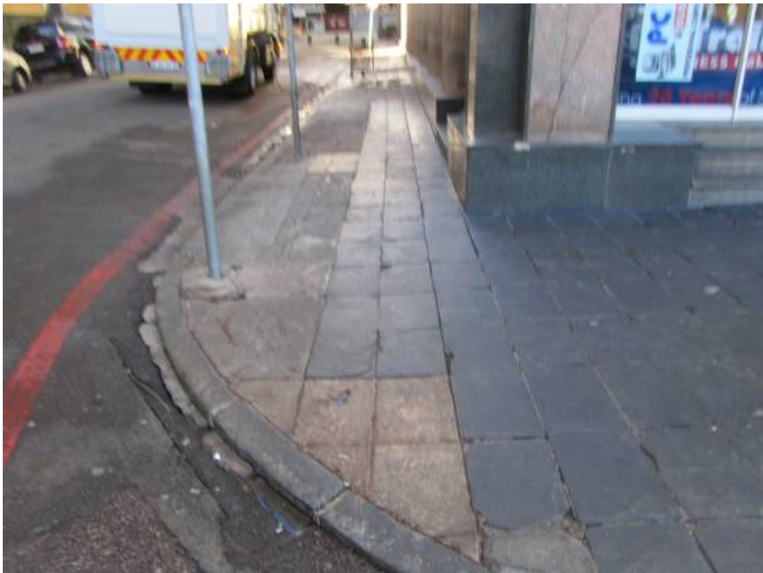
Figure 171. Although some historical slate survives the general condition of this section is not satisfactory. (P 974).
