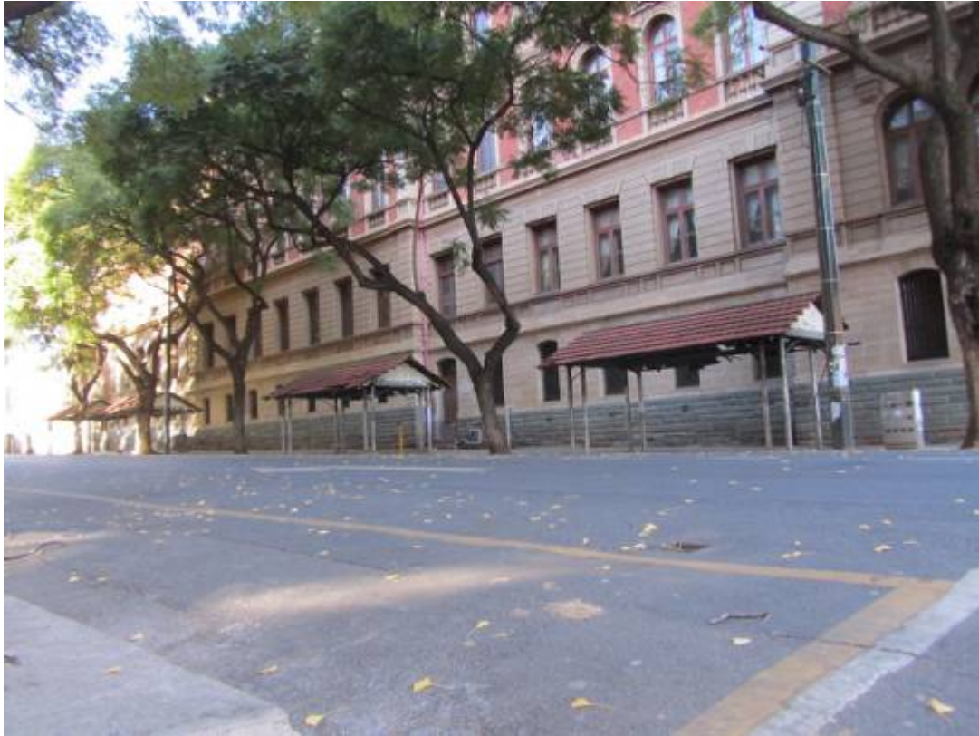
Figure 125. Protected historic bus shelters in need of repair. (P 925).
