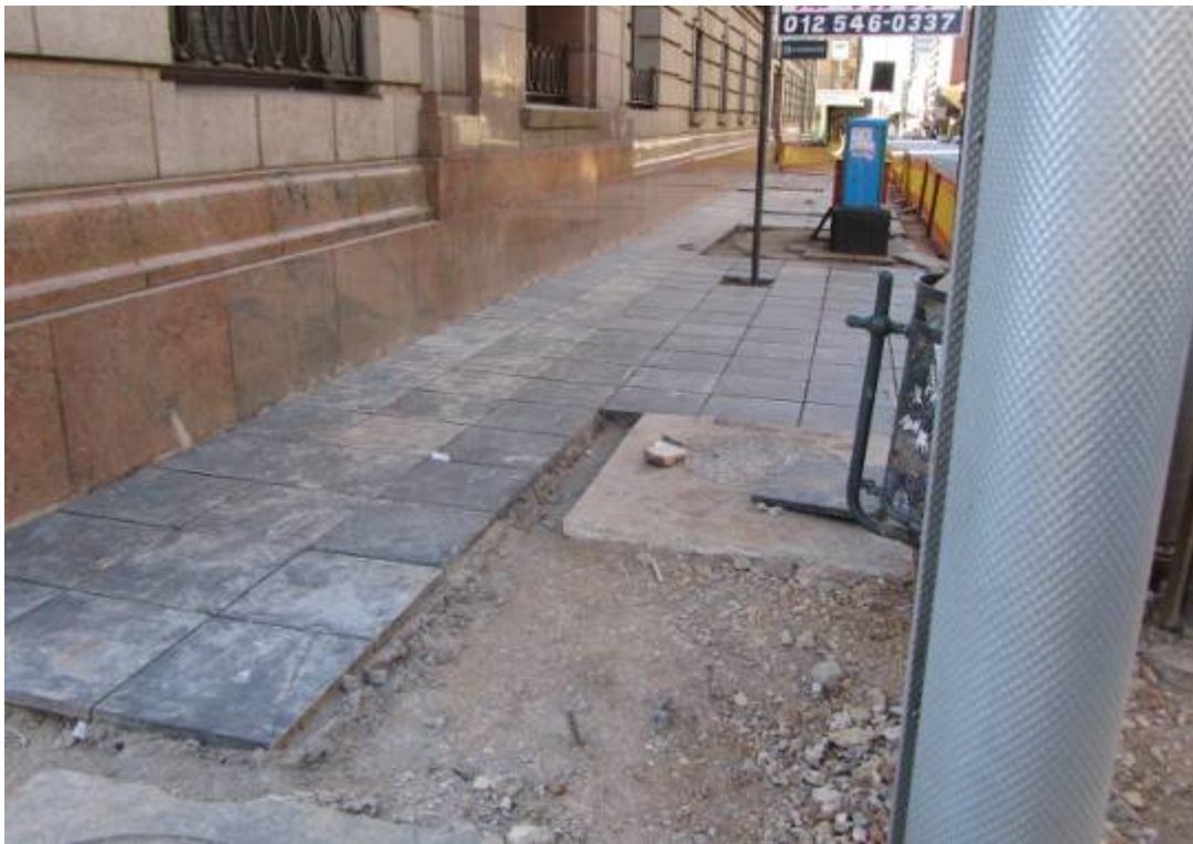
Figure 205. Historical (?) paving r- instated. whether this is the old slate that was re-sized in unknown.. NOTE:- Matter to be investigated. (P 1007).
