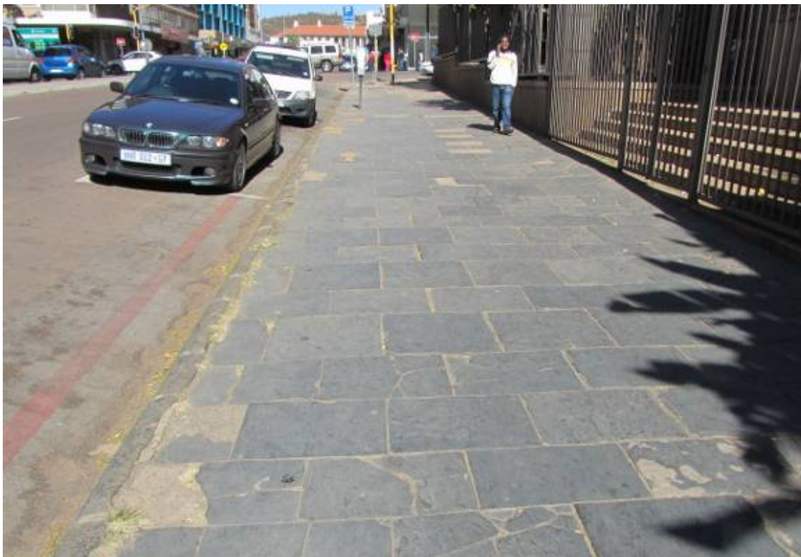
Figure 304. Protected paving. Repair necessary. (P 1132)
