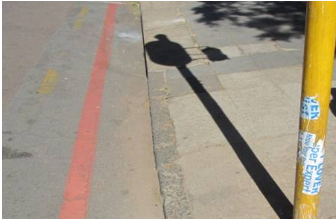
Figure 297. Granite curbing nearly covered by continuous re-surfacing. (P 1122)
