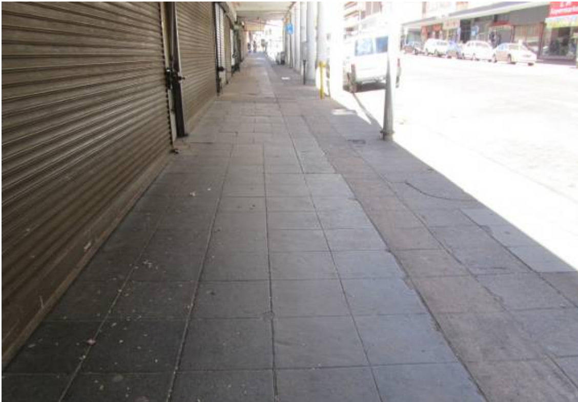
Figure 233. Cement block paving, remnants of historical slate paving and granite curbing defining old roadway. (P 1032)
