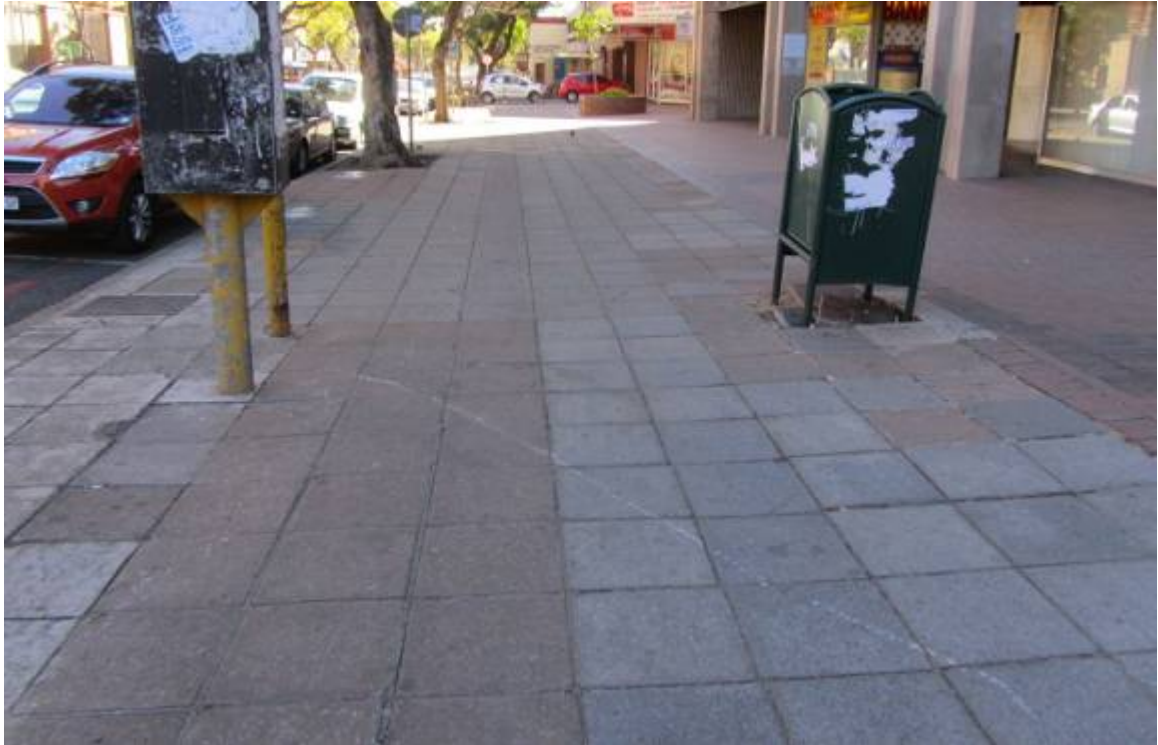
Figure 112. ‘The concrete block here demonstrates its adaptability to accommodate services. In the long term it will be preferred if the blocks are standardized (P 911).
