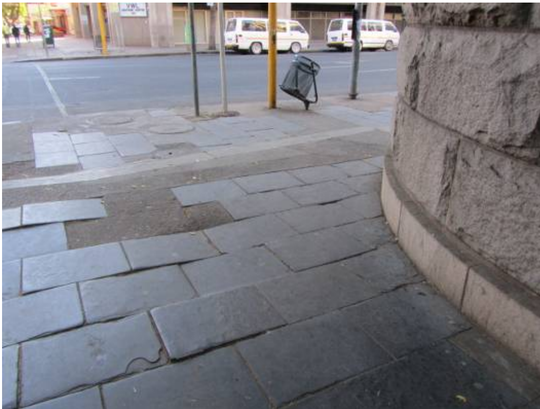
Figure 122. Historical slate paving adjacent to historical building. Note discontinuation owing to services and unsafe surface. (P 921).
