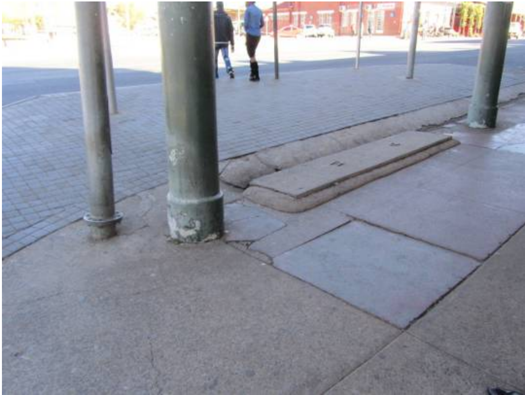
Figure 329. Roadway, sidewalk level irregularities. (P 1102)
