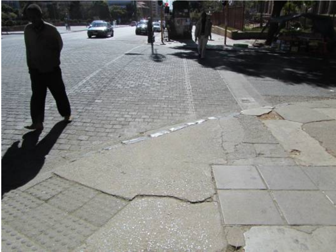
Figure 293. New road paving as part of 'Museum walk' renovation several years ago. Paving in view not repaired. (P 1118)
