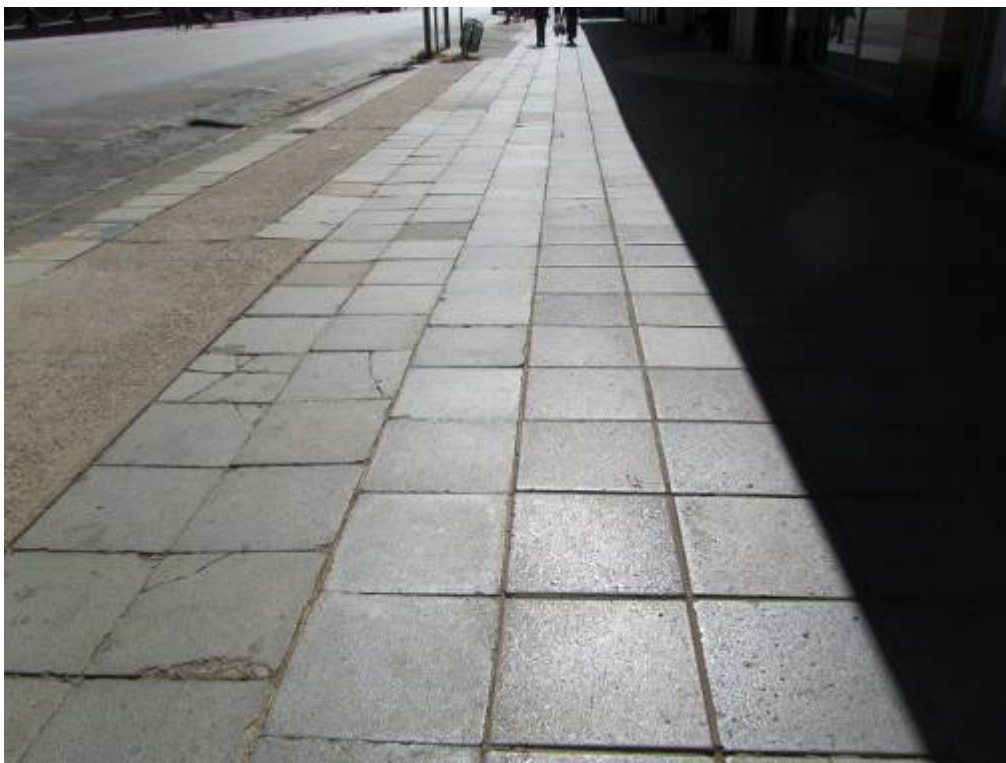
Figures 279 and 280. This earlier type of cement block pavers can be attractive if uniformly laid to a design. There should be a 'repair policy for paving after service trenching and reinstatement. (P 1080 and (P 1081).
