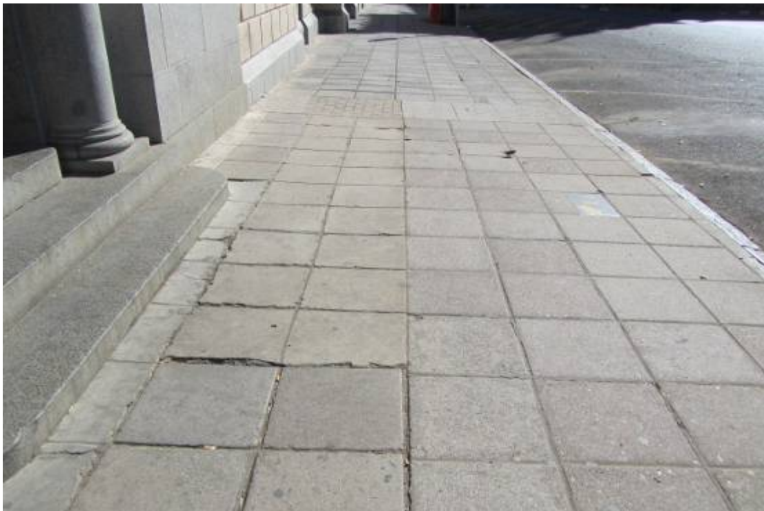
Figure 200. Large cement blocks as paving adjacent to historical building. Granite curbing stones defines sidewalk limit. If paving is used to retain character then the buildings should be investigated to define paving. (P 1003).
