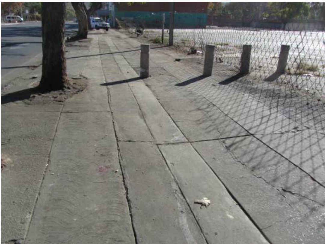
Figure 41. Modern sidewalk. Services issue apparent. (P818)
