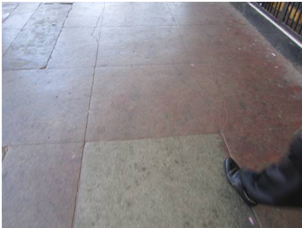
Figure 328. Detail of ferro-granolite panes and repairs. (P 1101)
