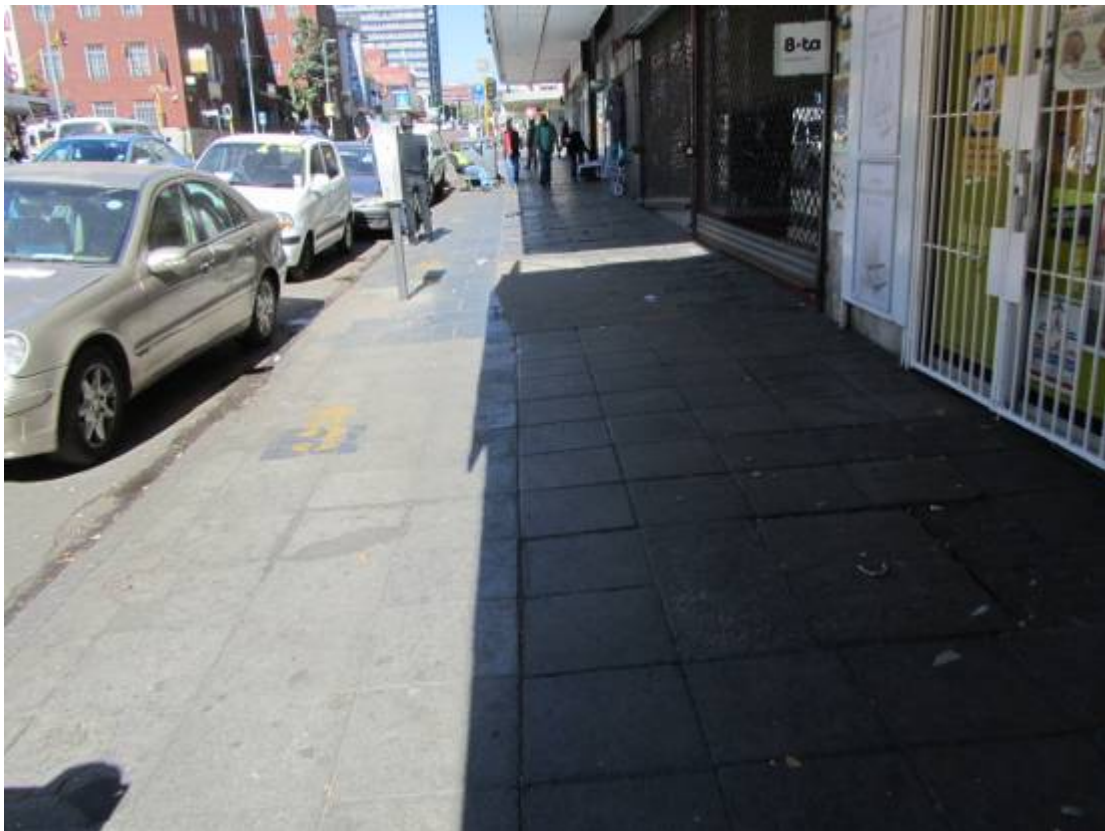
Figure 222. Cement block paving, remnants of historical slate paving and granite curbing defining old roadway. (P 1022)
