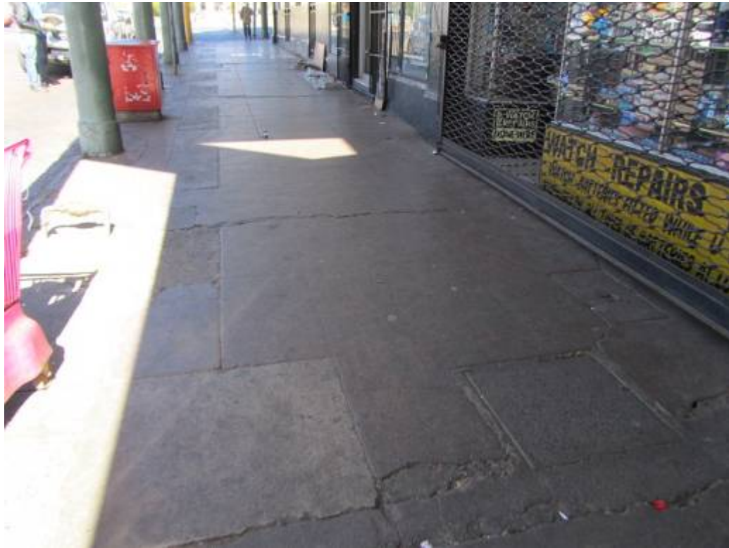
Figure 327. These ferro-granolite concrete panels may be indicative of historic paving. Similar panels were found in earlier blocks. Unfortunately they were also damaged and badly repaired over time. (P 1100)
