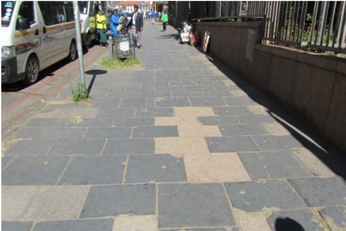
Figure 303. Protected paving. Repair necessary. (P 1131)
