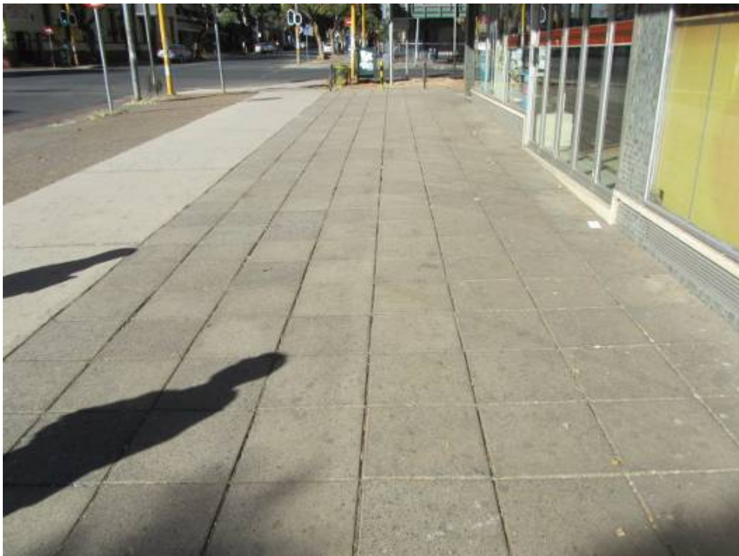
Figure 77. Strip concrete and bare earth sidewalk complemented with mid to later twentieth century square paving blocks. These paving blocks are practical and may be successfully re-applied in other areas. (P 863)
