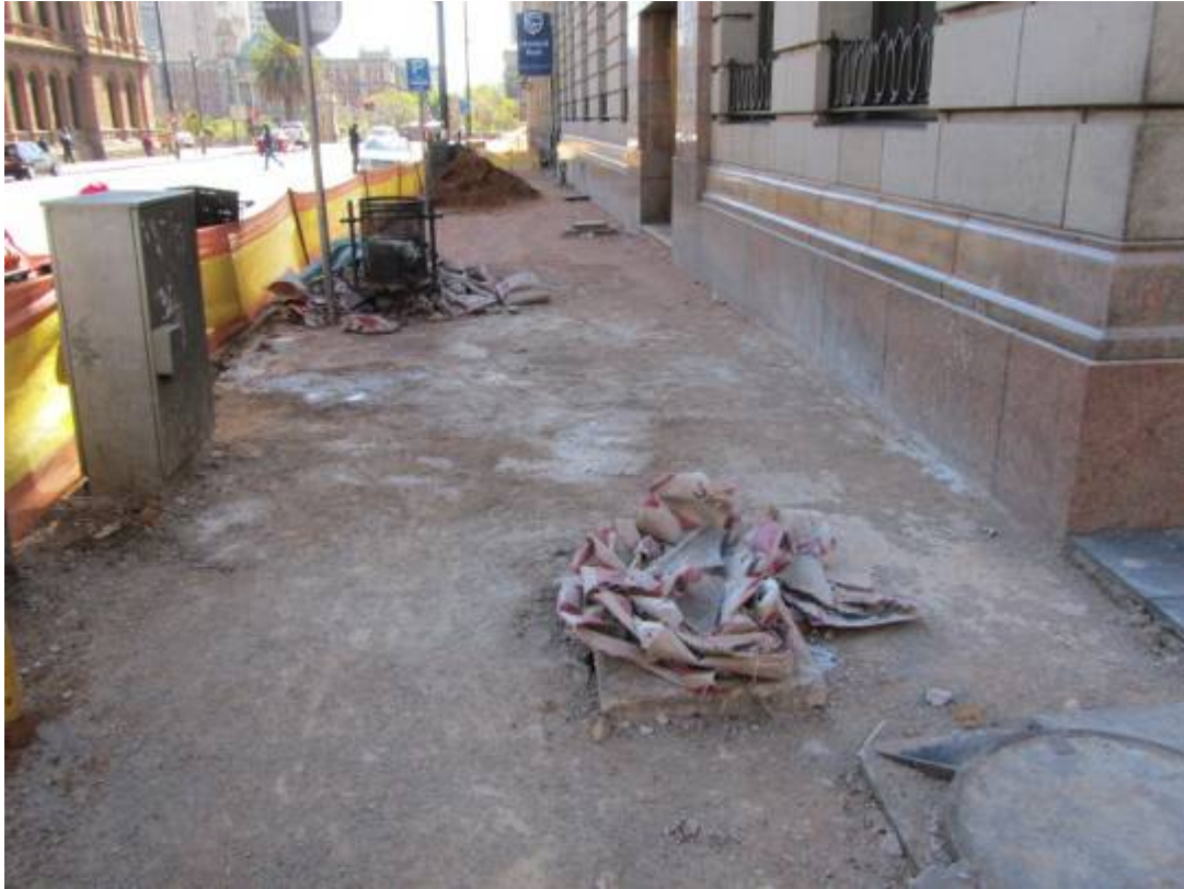
Figure 204. Historical slate paving being lifted adjacent to historical building. Note that no excavations were undertaken to alter paving level. (P 1006).
