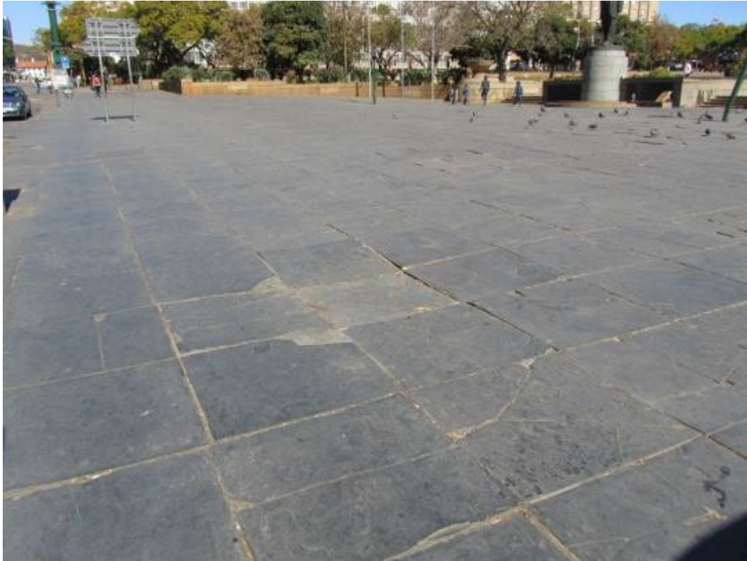
Figure 290. Protected paving. Repair only where public safety requires. (P 1087)
