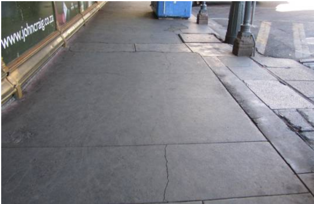
Figure 163. The paving adjacent to this historical building is a dog's breakfast of cement and concrete. The main problem with large areas of concrete is always unsightly cracking. With blocks or paving bricks this can easily be remedied. (P 966).
