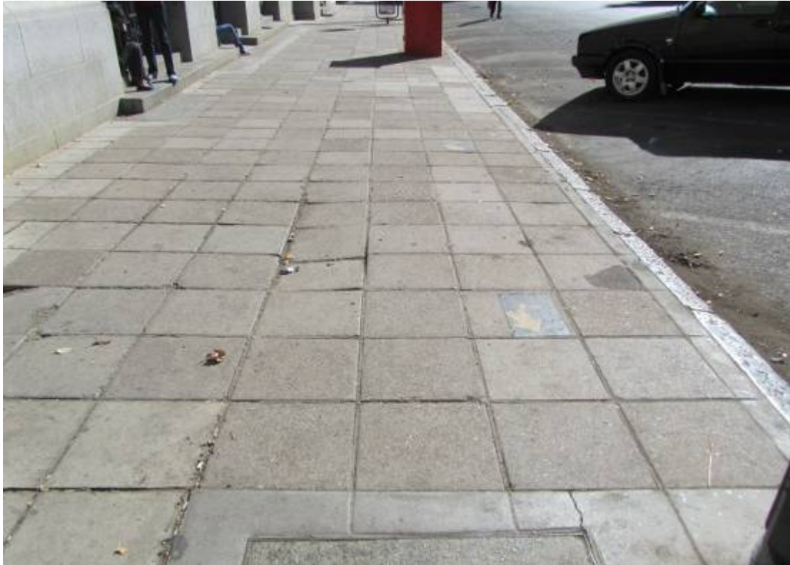
Figure 199. Large cement blocks as paving adjacent to historical building. Granite curbing stones defines sidewalk limit. (P 1002).
