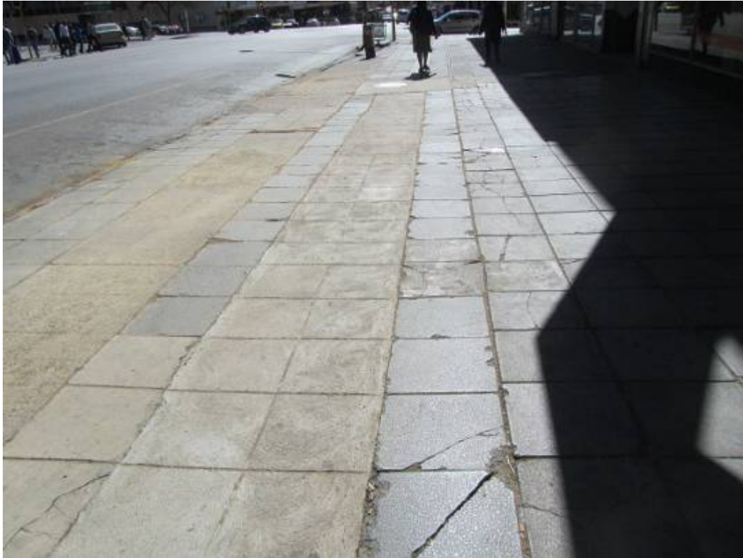
Figure 265. Variety of paving materials. Note that some worker in the past tried to make the strip concrete match the paving blocks. (P 1062)
