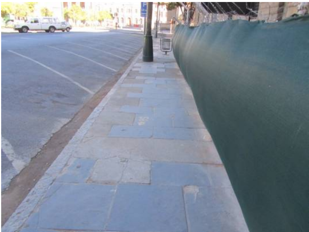
Figure 148. Original slate paving adjacent to historical building Construction in progress without protection. (P 951).
