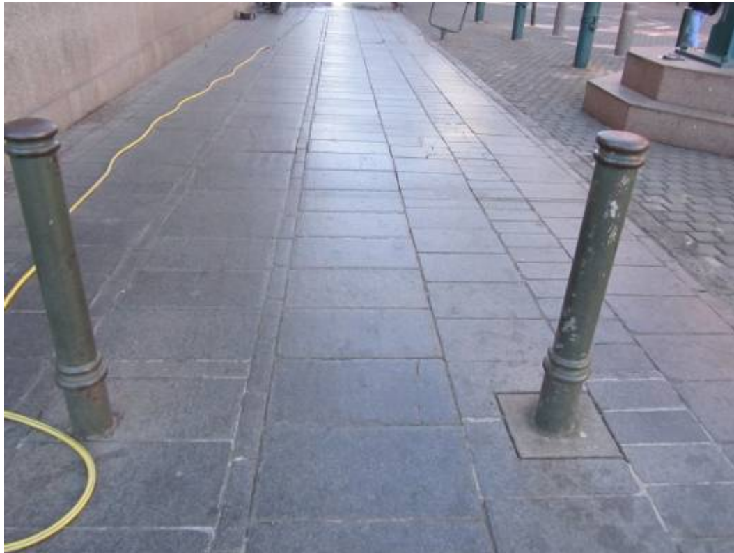
Figure 159. The refurbished paving in the Church Street Boulevard is excellent and may well become the type pattern for the present project. (P 962).
