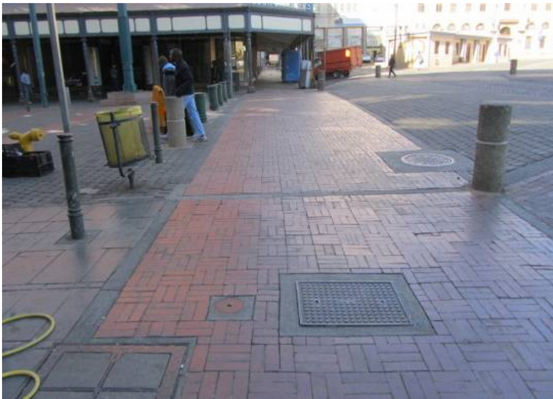
Figure 158. Mixed new paving at Church Street pedestrian boulevard. Note marked difference in road level. Service access-covers well blended as features rather than eye-sore. . (P 961)
