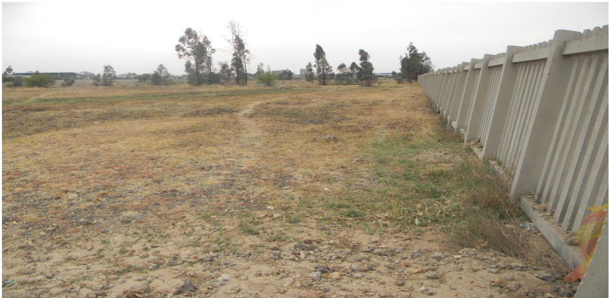
Plates 3: Shows section of fence to be removed. Note that the fence is already collapsing, either way, the fence will still need to be rehabilitated.
