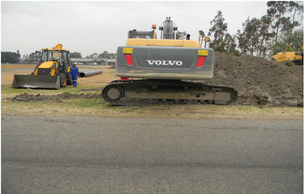
Plate 12: Shows excavators, note the size of the machines. They require more working space.
