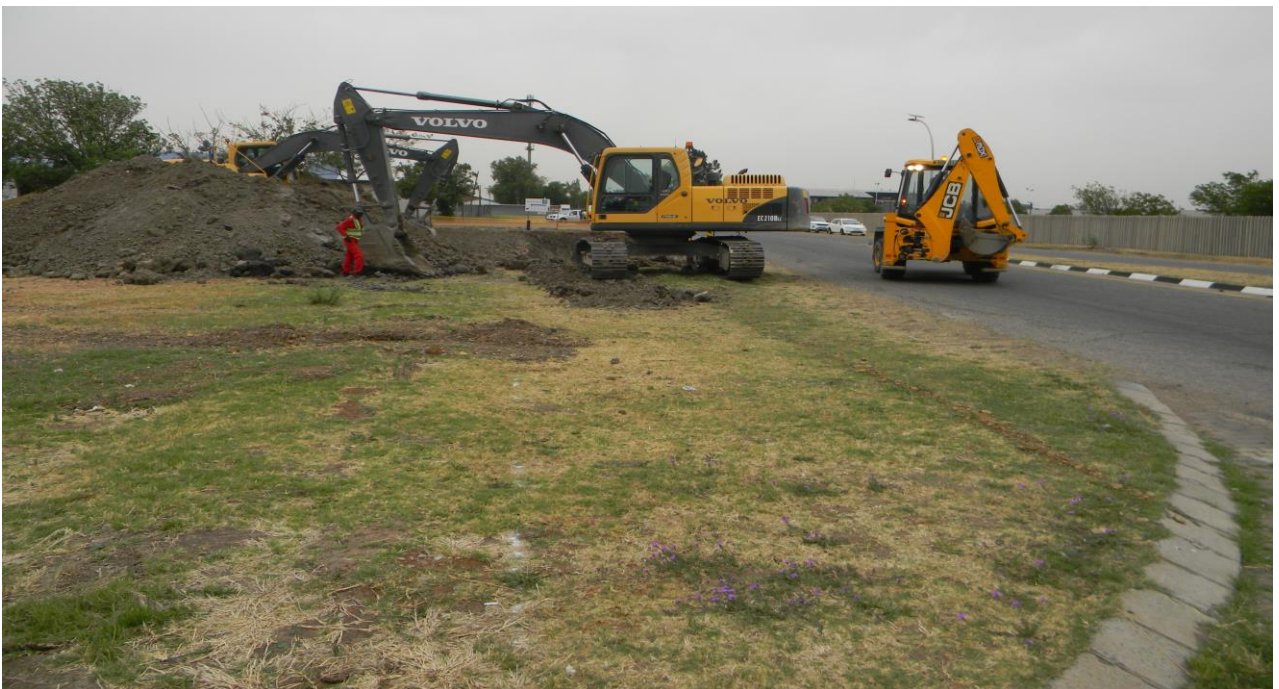
Plate 11: Shows excavators at work, note the size of the excavator requiring more 40m radius to turn.
