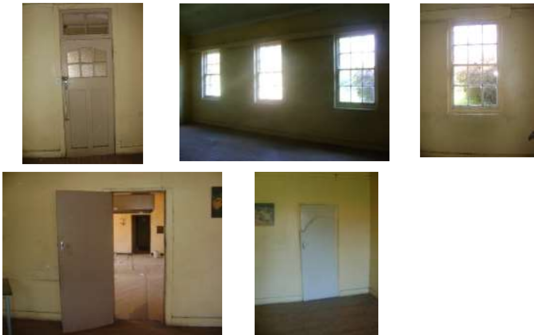
Figs. 92 to 96. Above are door and window details of room 8 in drawing 3. (Photographs, S.M. Miller 2016.)
