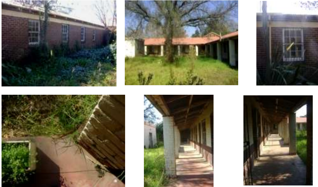
Figs. 127 to 132. Above are exterior elevations of rooms 18 to 24 in drawing 4. (Photographs, S.M. Miller 2016.)
