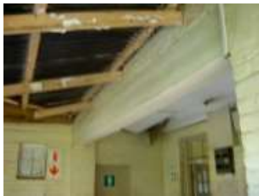
Figs. 241 to 247. Above is detail regarding the building in drawing ten. (Photographs, S.M. Miller 2016.)
