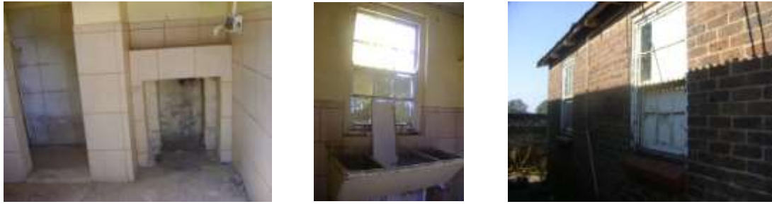
Figs. 287 to 289. Above is specific detail of buildings in drawing thirteen. (Photographs, S.M. Miller 2016.)
