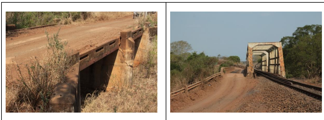
Fig. 8. Concrete road bridge near the railway line and an example where they share the same substructure.
