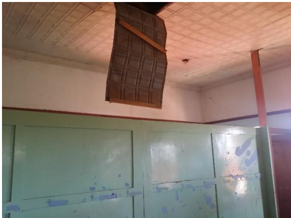
Interior: Pressed ceilings damaged by moisture and thieves
