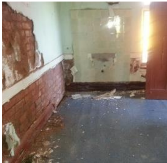
Interior: Damaged plaster
