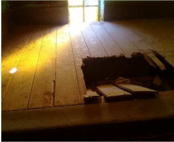
Interior: Damaged wooden floors
