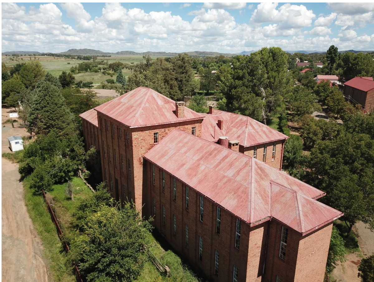
Exterior: North West aerial elevation indicating roof that requires attention
