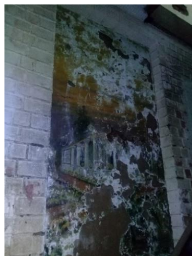
Interior: Murals damaged by moisture
