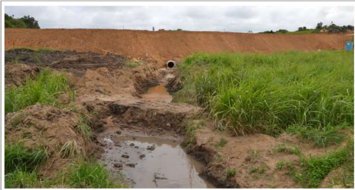
Photo 5: State of the stream channel passing under the recently realigned road south of the proposed quarry
