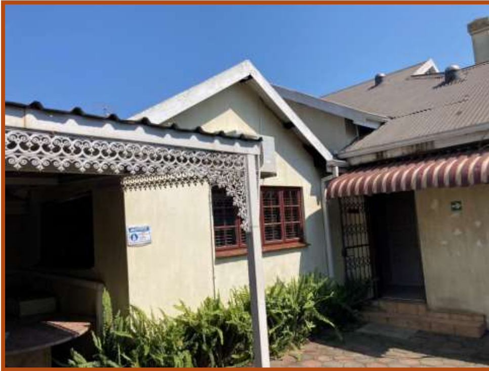
Figure 13: Notice the intricate architectural detail portrayed on the image. Firstly, take note of the roof vents close to the chimney and gable. The architect put emphasis on proper ventilation of the house because of the corrugated iron roof although the vents may also have served for decorative purposes. Shifting to the veranda, pay attention to the decorative laces. These were also a key facet of Victorian architecture and were intended for decorative purposes.
