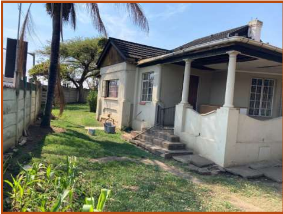
Figure 8: A closer view of the property showing the overall outlook of the building. Note the wooden cladding on the gable suggesting some additions to the building at some point.
