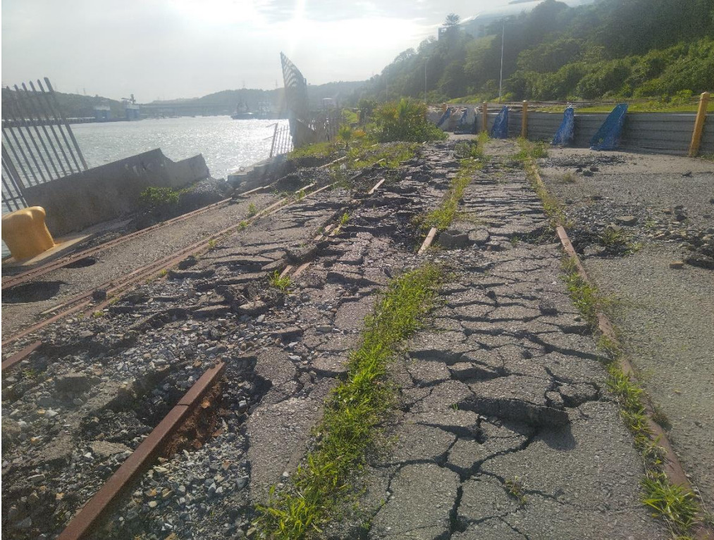
Figure 1: View of the collapsed ferry landing
