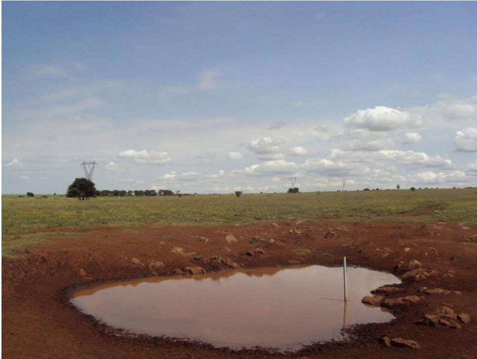
Figure 4: View showing excavation for livestock waterhole on the west section of the project footprint
