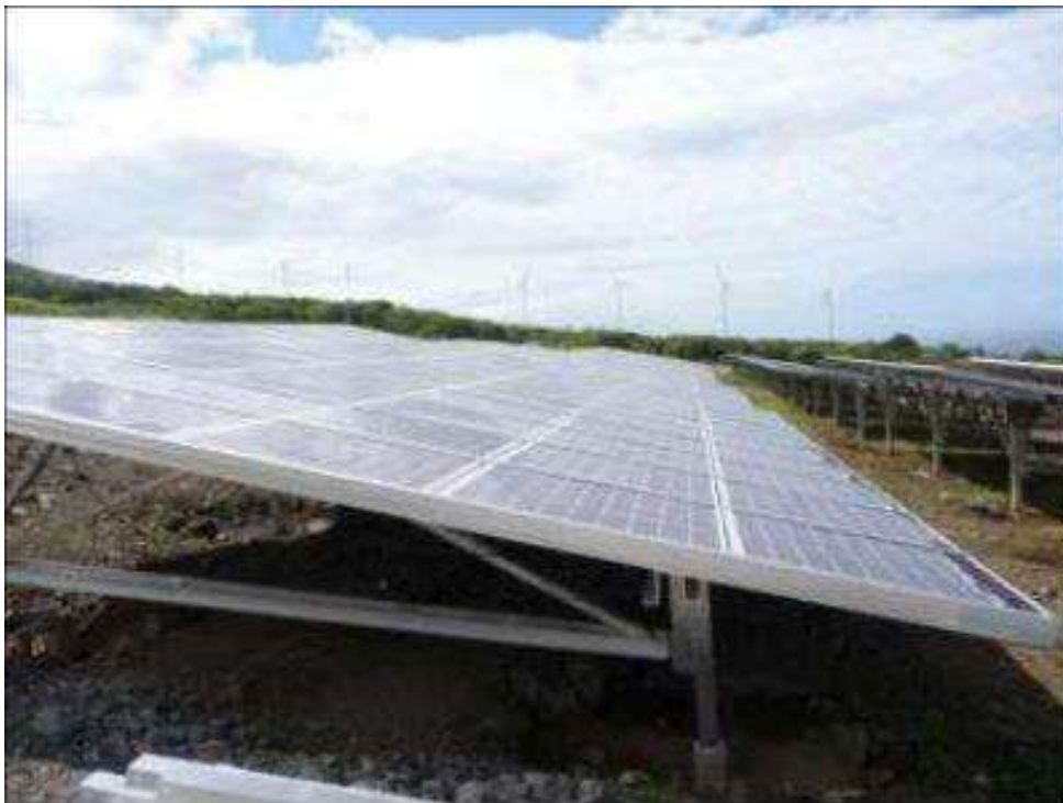
Figure 19: Example of Fixed Solar Panels (Nemai 2023)
