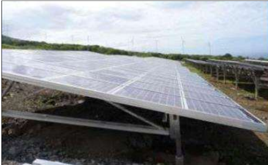
Figure 14: Example of Fixed Solar Panels (Nemai 2023)
