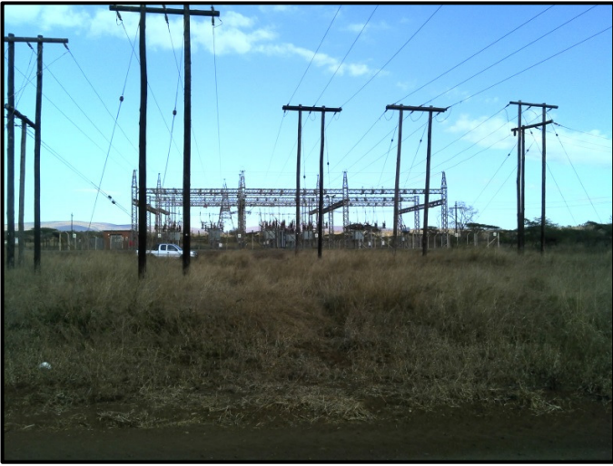
Figure 4. Existing substation for connection.
