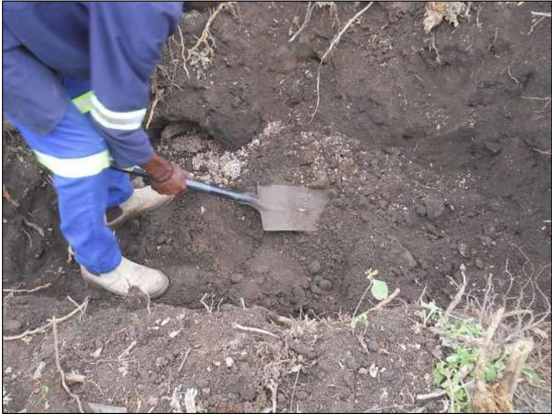
Figure 23. The test trench being extended. Note exposure of the termite nest above the shovel handle.
