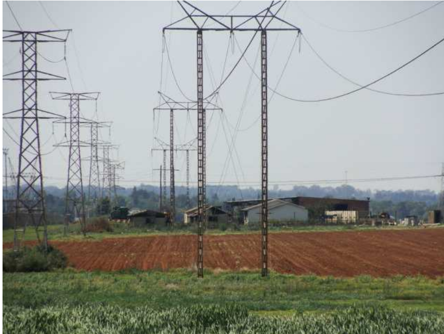
Figure 11 View along route alternatives 1, 2 and 4 across wetland area, towards the Kookfontein substation.
