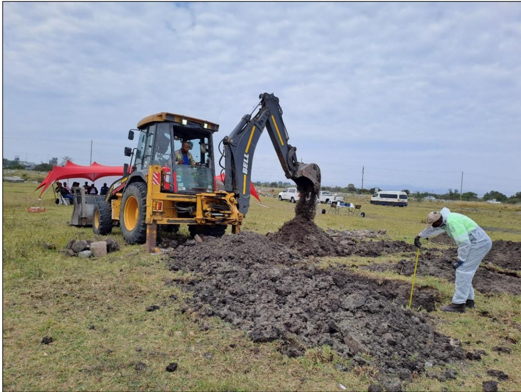
Figure 11 - TLB assisting with the exhumations on site with the guidance and monitoring from PGS.
