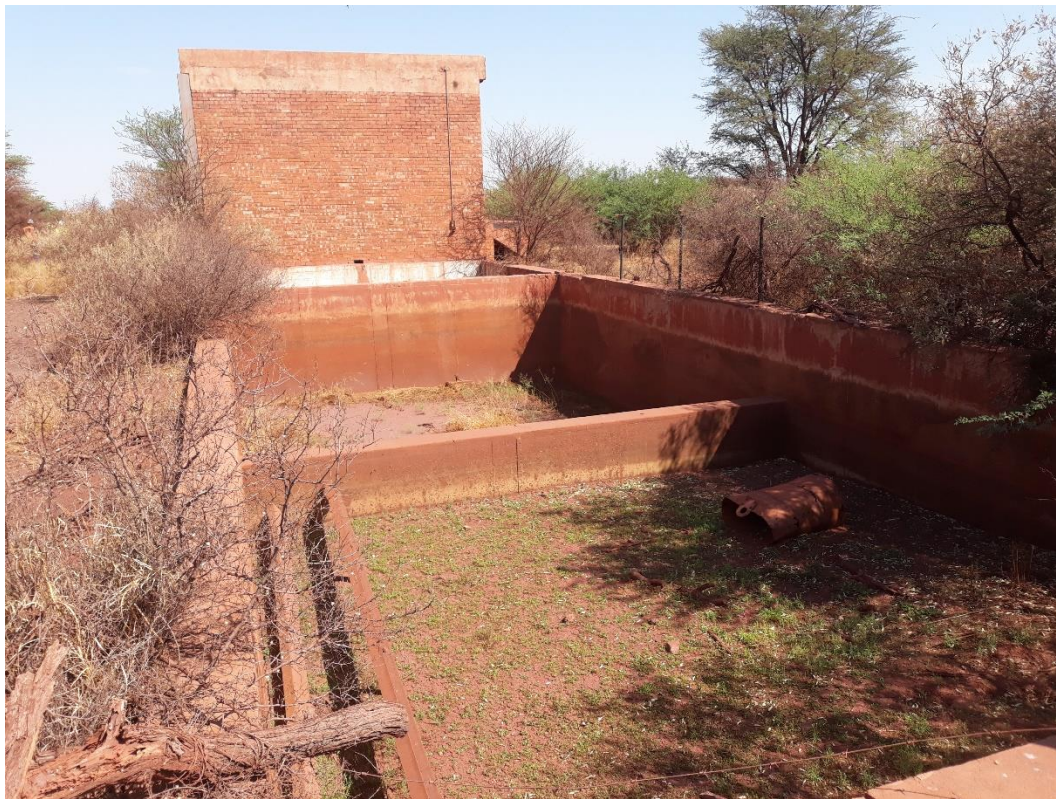
Figs. 26 to 28. Typical views of remaining walls of the settlement tanks. All equipment has been removed and buildings have been vandalised. They have no heritage value. (Photos S.M. Miller 2020.)
