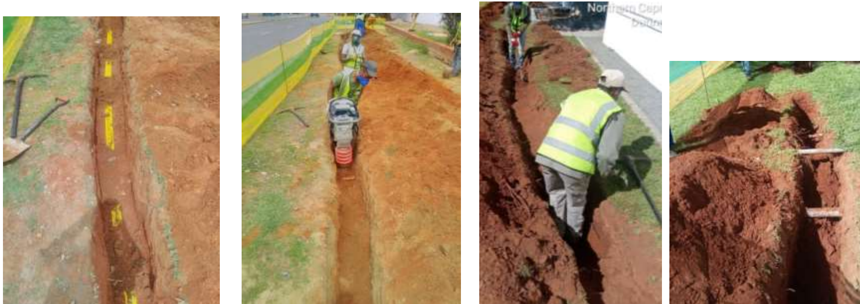
Figures 3 - 6: Some photographs of conventional trenching within the Sol Plaatje Municipal area
