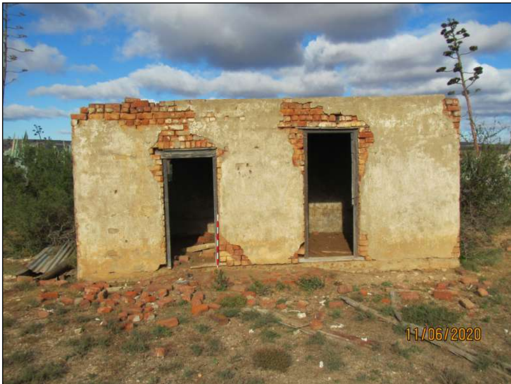
Figure 31 - A dilapidated brick labourer house was found on the farm Britzkraal 253 (SF-09). The windows and doors of the house have been removed, and the house has been abandoned.
