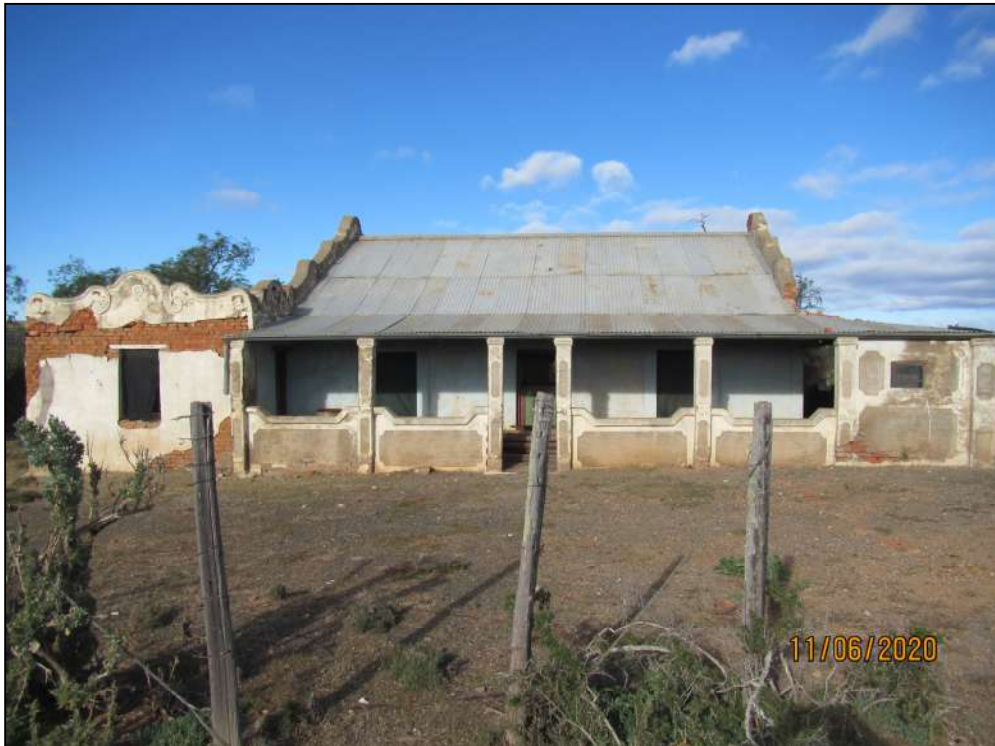
Figure 25 - A dilapidated house with a small outbuilding was found on the farm Britzkraal 253.
