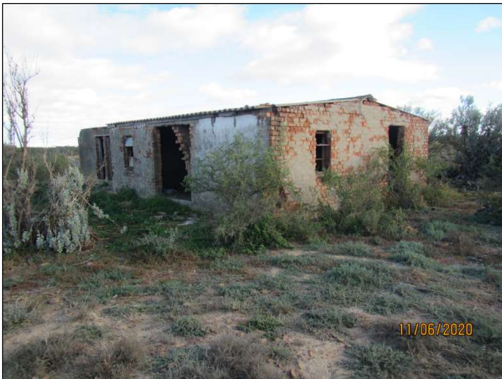
Figure 29 - A dilapidated brick house was found on the farm Britzkraal 253 (SF-08). The windows and doors of the house have been removed, and the house has been abandoned.
