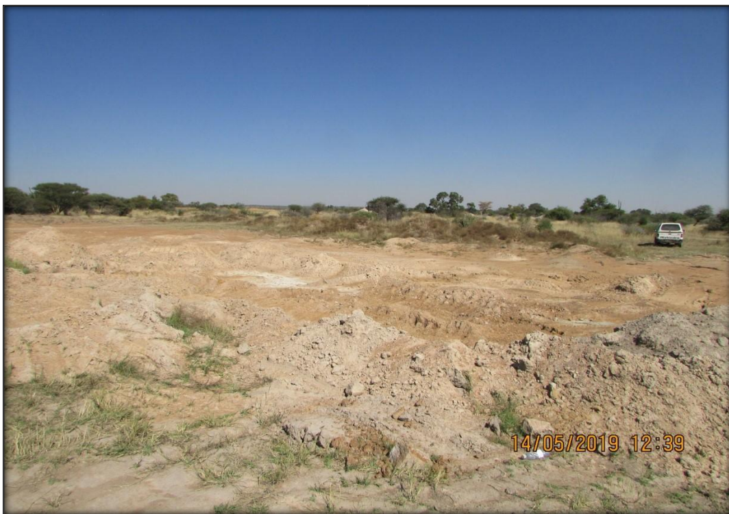
Figure 7: A view of the sand quarrying in the area. This shows only a small section.
