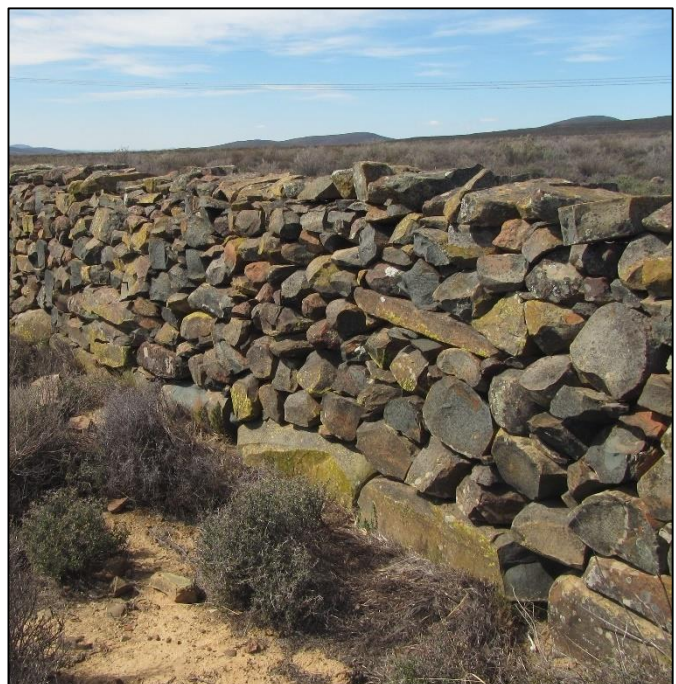
Figure 13: View of the wall where the full height is preserved. The cap stone slabs are visible on the top (waypoint 079).
