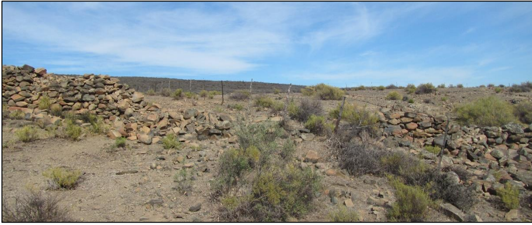
Figure 21: View towards the west-southwest showing the place where the stone walling has been demolished to ground level to allow for the erection of a wire fence (waypoint 068). This is the point through which the new road will now pass.
