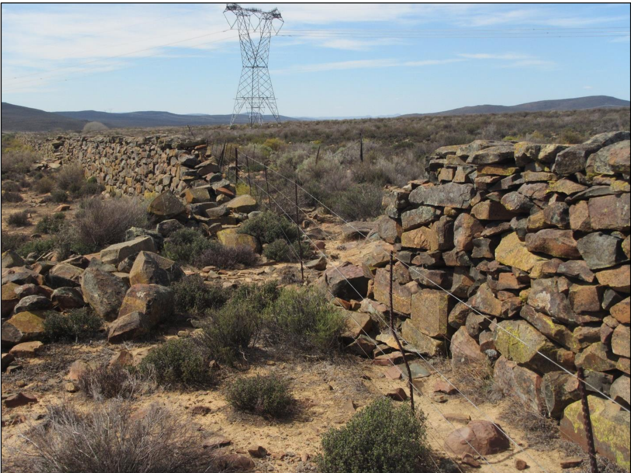
View towards the east showing a place at waypoint 080 where the wall has been demolished to facilitate wire fence construction.
