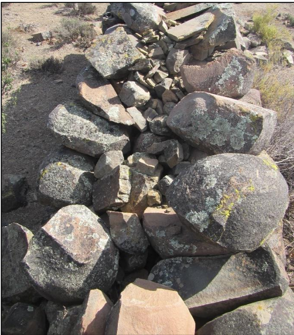
Figure 12: View of the top of the wall where the capping slabs are missing and showing the 'rubble fill between the two stone 'skins' (waypoint 067).
