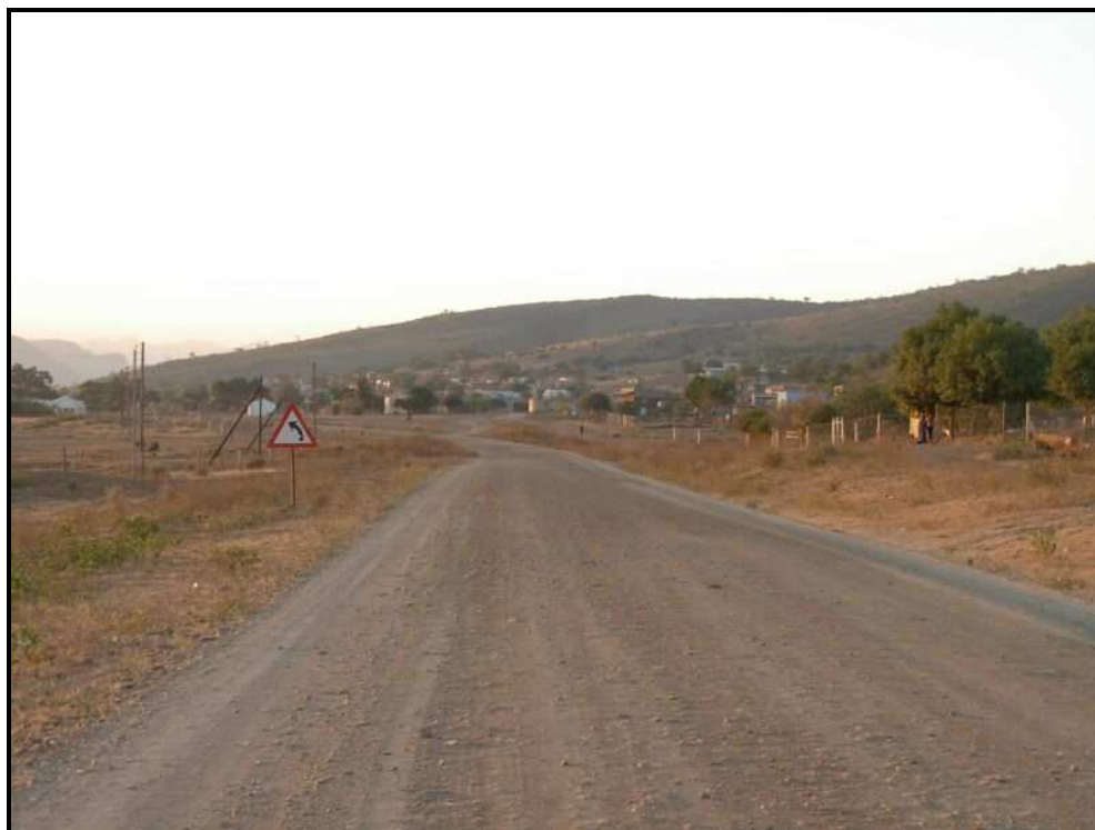
Figure 2: Road conditions close to Malokele
