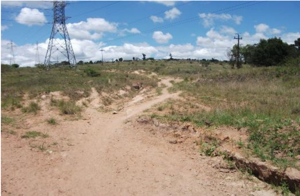
Figure 6: Eroded area with power lines
