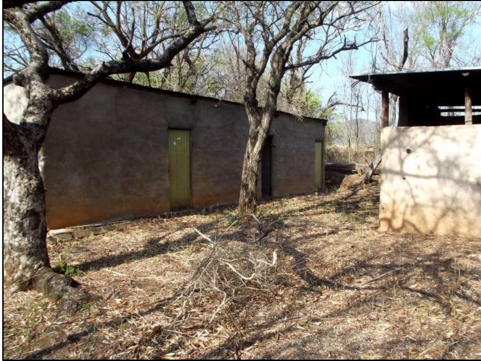
Figure 3. Site STR 3. Some staff quarters located close to site STR 1. They are currently not in use. The photo was taken in a South-Western direction.
