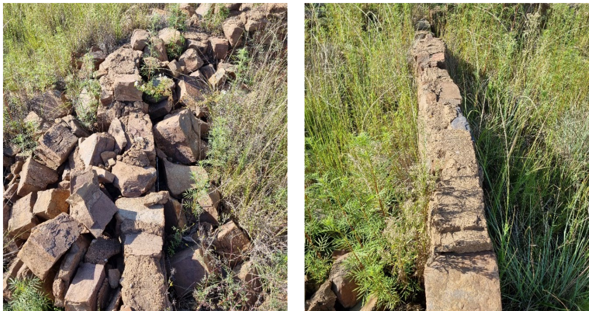
Figure 25: Collapsed free standing brick and cement walls. UP-DRB-2529-06 (left) and UP-DRB-2529-07 (right).
