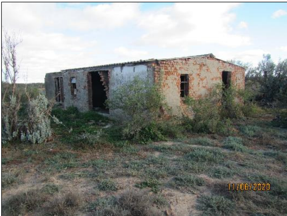
Figure 29 - A dilapidated brick house was found on the farm Britzkraal 253 (SF-08). The windows and doors of the house have been removed, and the house has been abandoned.
