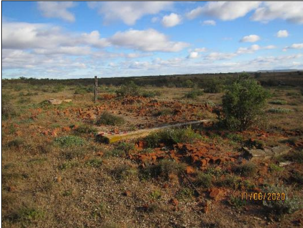
Figure 28 - The ruins of an old stable were found on the farm Britzkraal 253 (SF-07). Only the ruined foundations remained.
