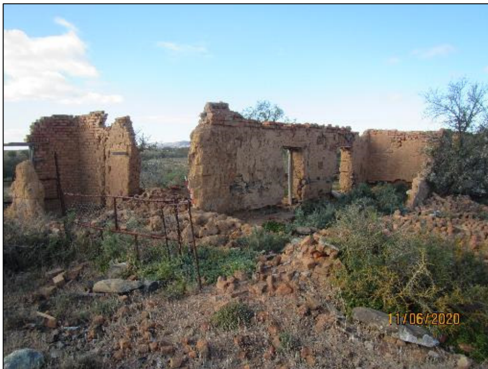
Figure 27 - A dilapidated brick house (SF-06) was found on the farm Britzkraal 253. The walls, windows, roof and doors of the house have been removed, and the house has been abandoned.
