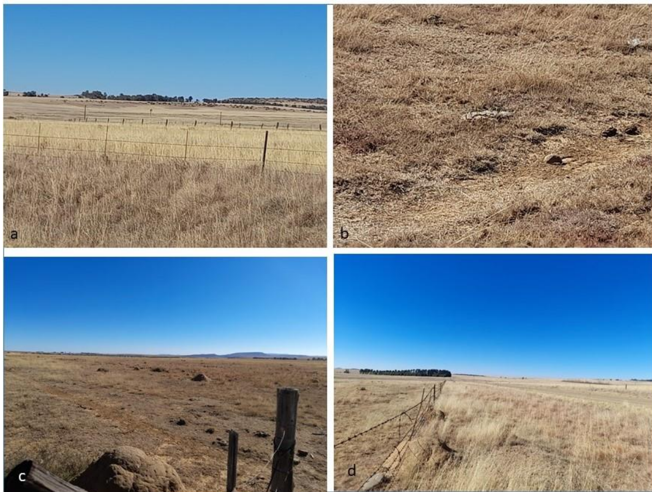
Figure 11: Rouxville to Zastron section starting north of Rouxville (see Fig. 5 for substation) where the new powerline crosses from the east side to the west side of the R26 road; Middelfontein; a – powerline comes from centre background to centre foreground in grassland; b – closeup of the soils and grasses showing no rocky outcrops; c – beginning of west side route in grassland with deep soils and termite mounds; d – route goes down the centre of the photo towards Zastron.
