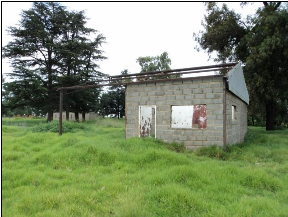
Figure 15: Dilapidated structure Alt 1.
