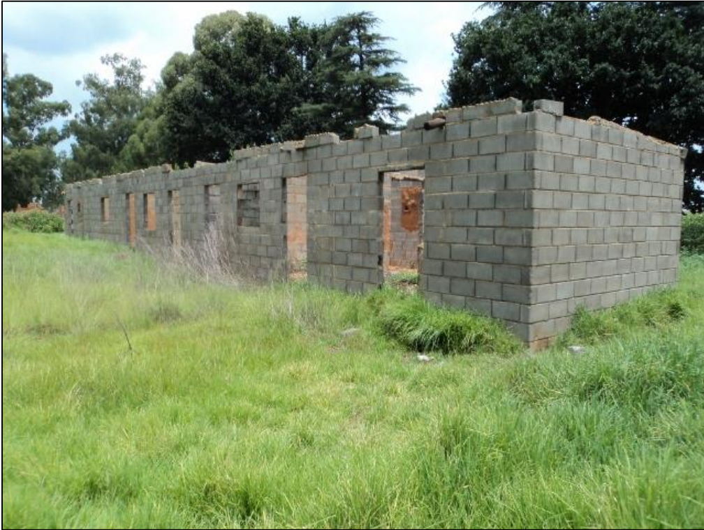
Figure 16: Dilapidated structure Alt 2.
