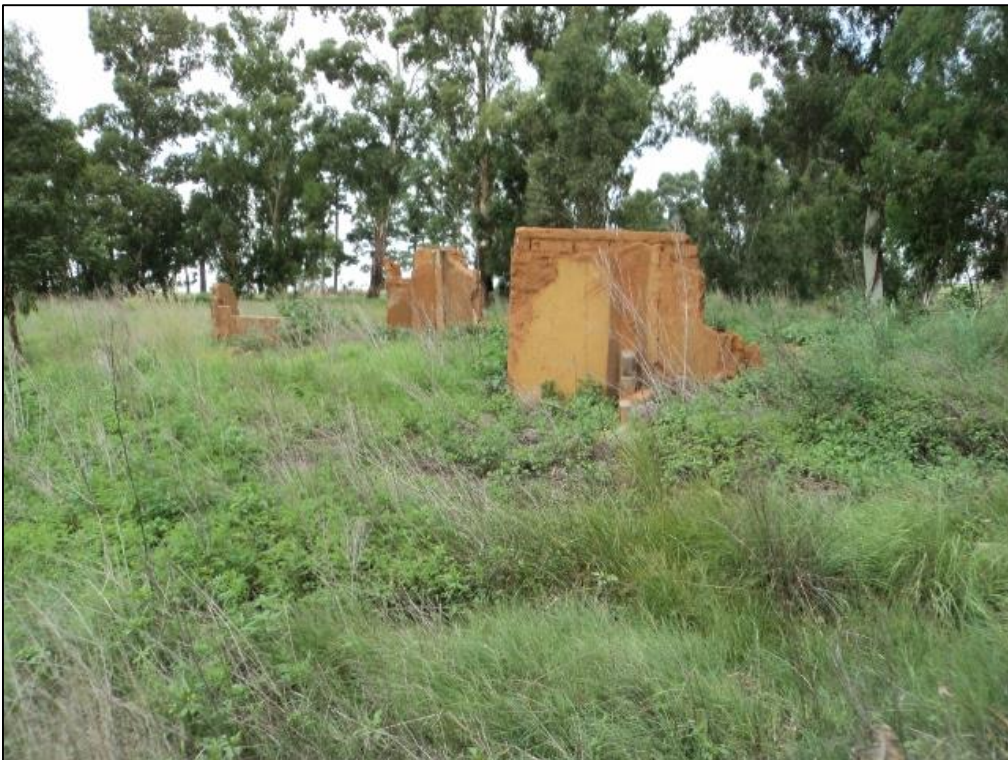
Figure 17: Dilapidated structure Alt 3.
