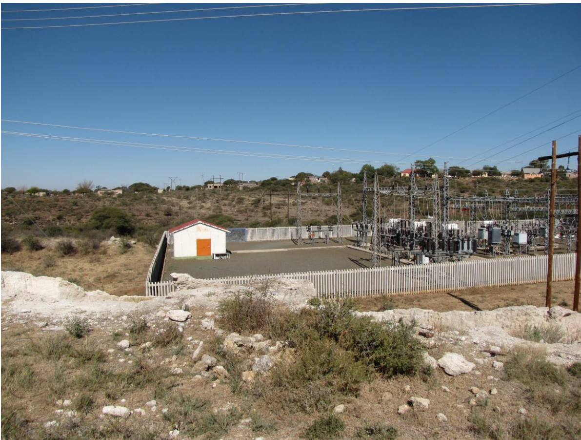
Figure 3: The Norlim Substation looking south (27°37.263' S, 24° 38.407 E')
