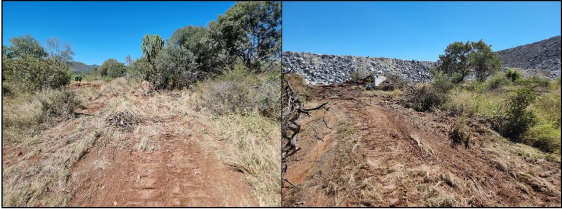
Figure 5-2: View of service roads constructed within a section of the project area.
