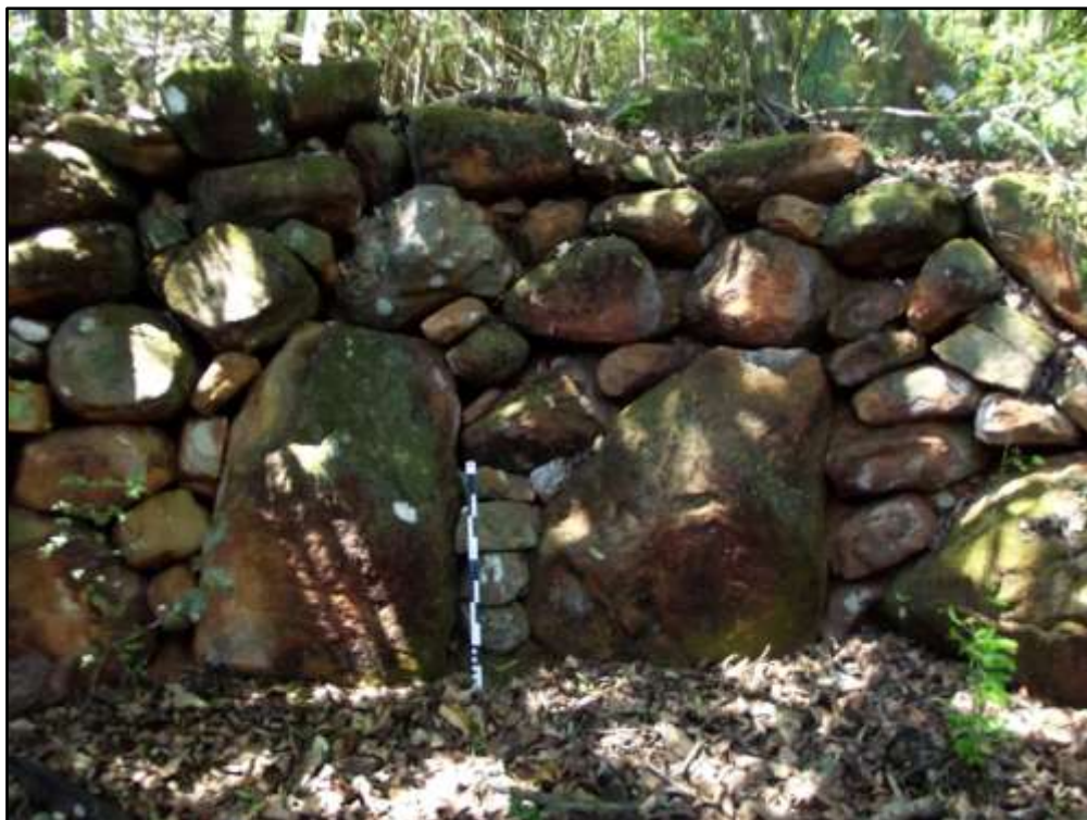
Figure 10. A photo of the inner side of the enclosure wall at site BL 4B.
