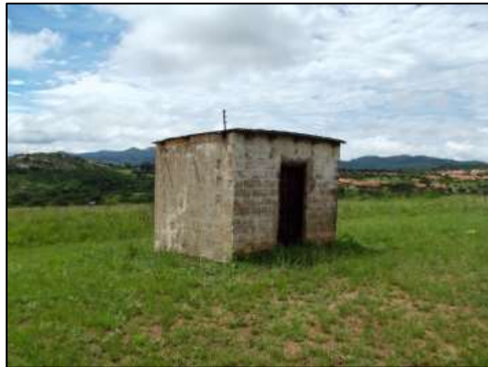
Fig. 2. Site TRB 2. The water pump facility. Photo taken in a southern direction.
