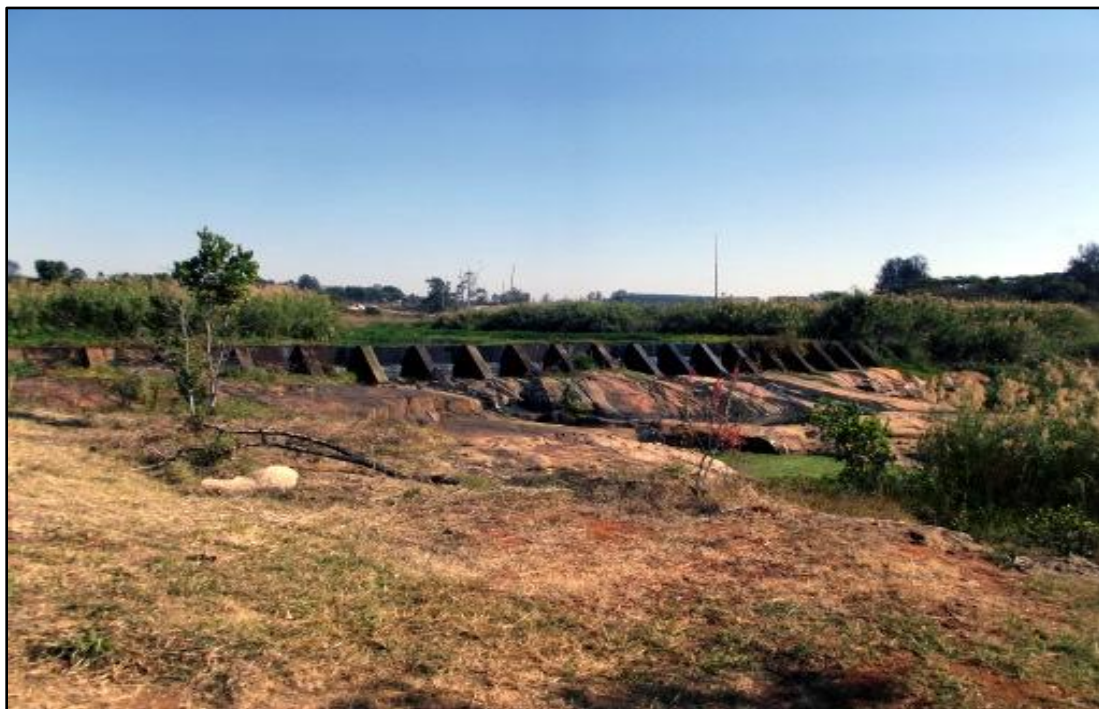
Fig. 18. Site WWA 6. The historic weir in the White River. Photo taken in south-western direction.
