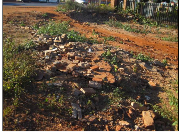
Figure 6: View of some of the rubble left on site after demolition of the buildings.
