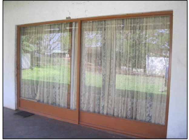
Figure 22: View of one of the metal framed doors of the house.
