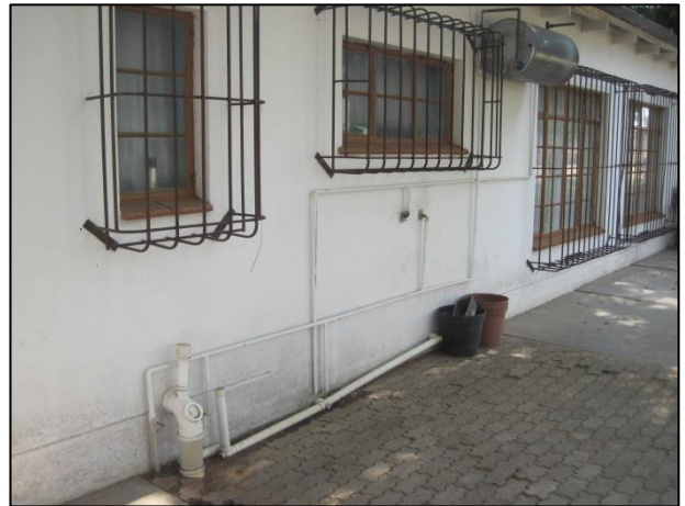
Figure 24: View of the external plumbing system of the house.
