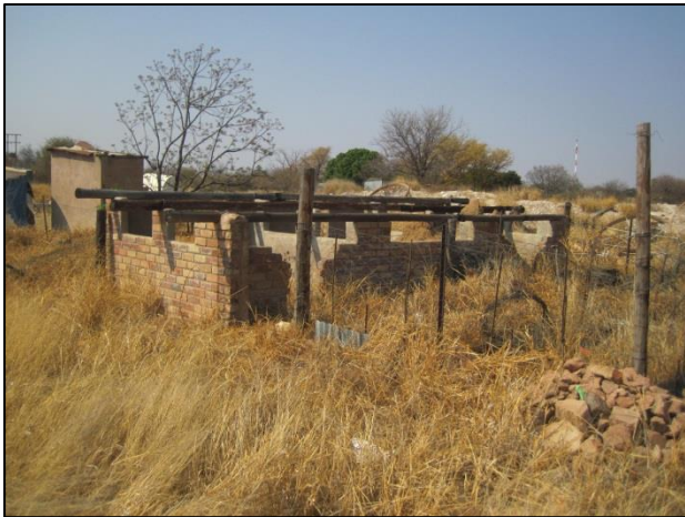
Figure 7: View of the dilapidated pigsty.
