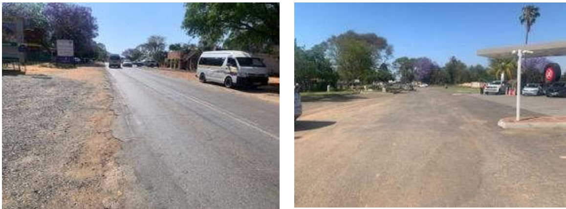
Figure 10 – Intersection C – Road Condition
