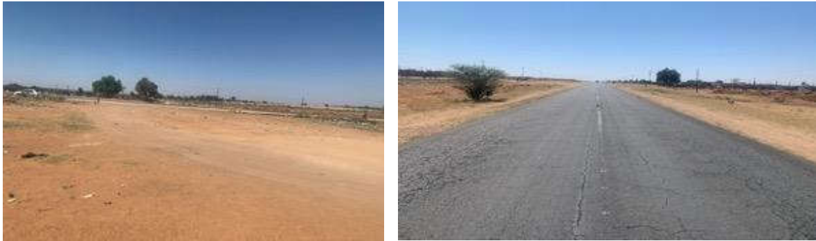
Figure 9 – Intersection C – Road Condition
