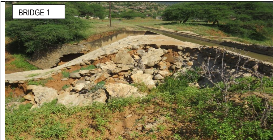
Figure 4: View of the dilapidated bridge one
